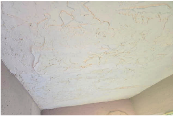
9 Unit 107 Bulging Stucco w/Water Staining on Patio Roof
