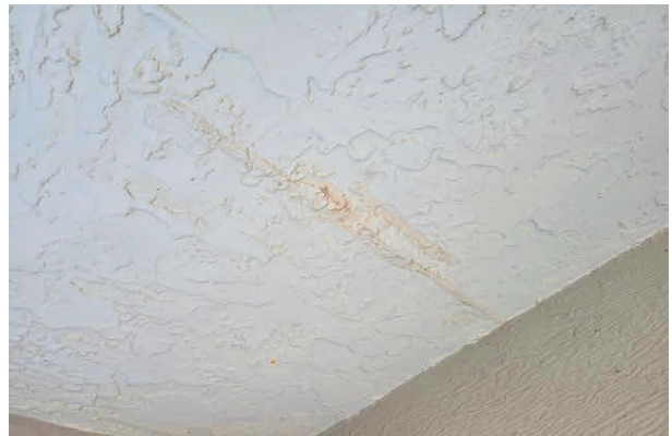
6 Unit 107 Bulging Stucco w/Water Staining on Patio Roof
