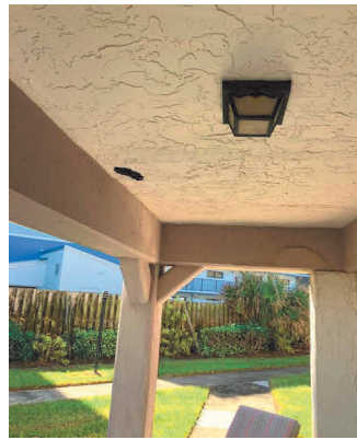
10 Unit 107 stucco removed
