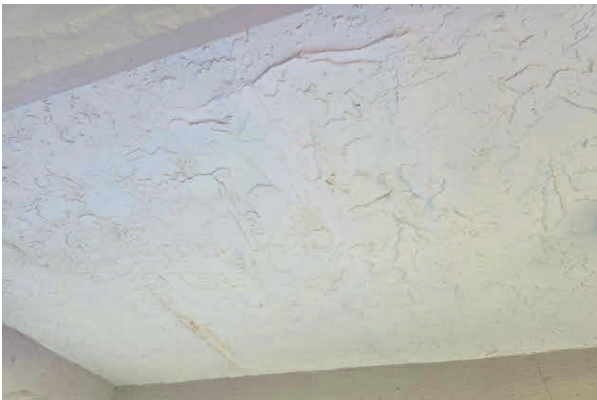
5 Unit 107 Bulging Stucco w/Water Staining on Patio Roof
