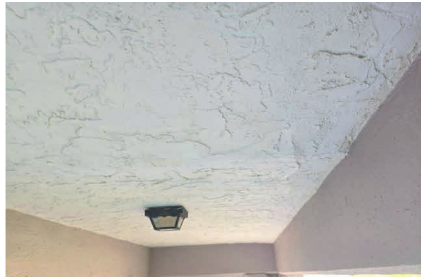
8 Unit 107 Bulging Stucco w/Water Staining on Patio Roof
