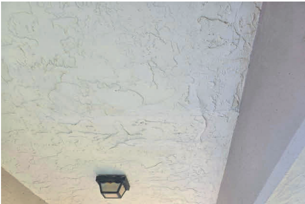
7 Unit 107 Bulging Stucco w/Water Staining on Patio Roof
