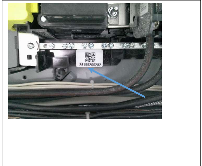
Manufacture Date for the electrical panel (2026)
