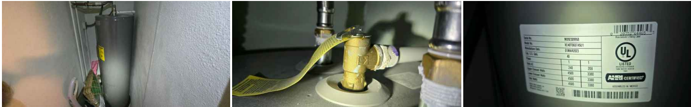
Under cabinet plumbing & drains
