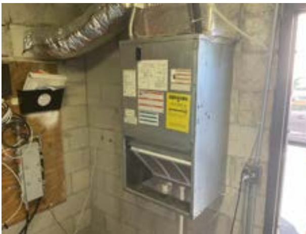
Air handling unit
