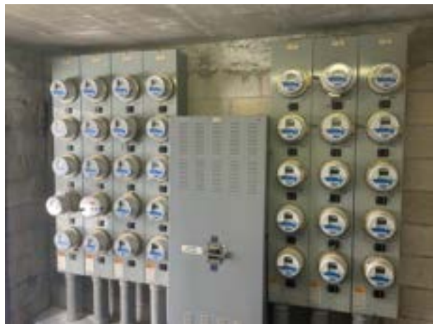
Electrical system components
