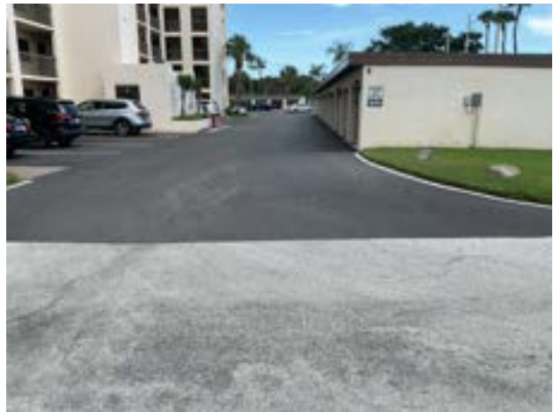
New vs old pavement
