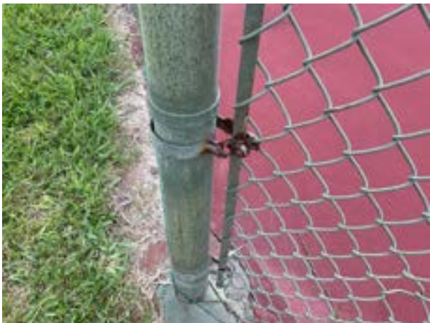
Broken fence link with rust
