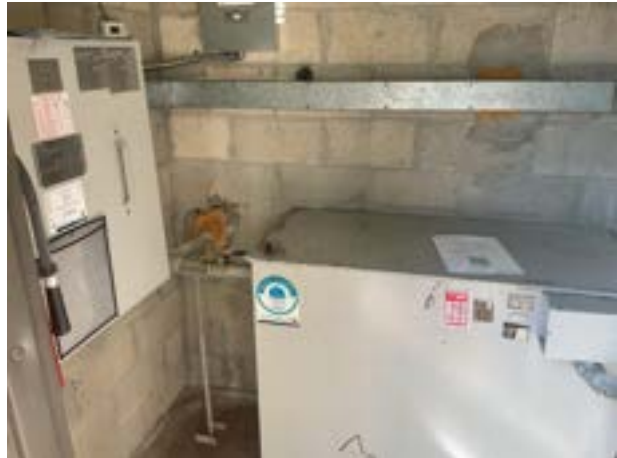
Building 10 elevator equipment
