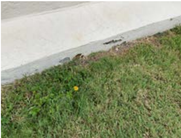
Deterioration at grade
