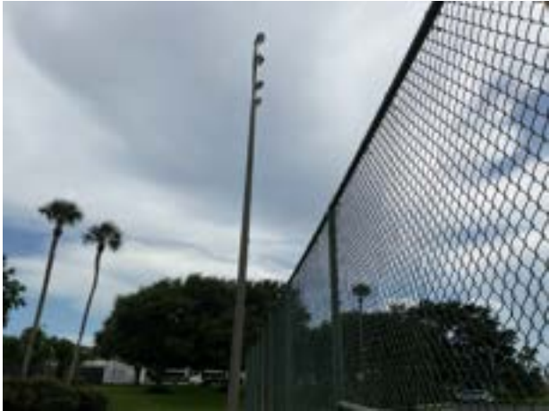
Light pole and fixture
