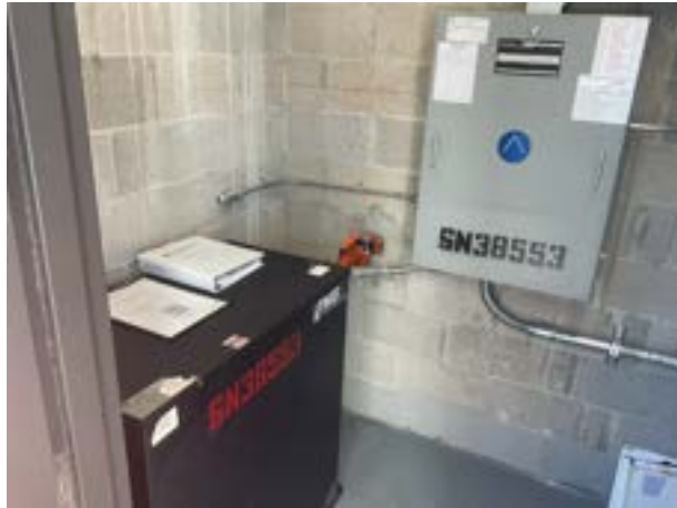
Building 9 elevator equipment
