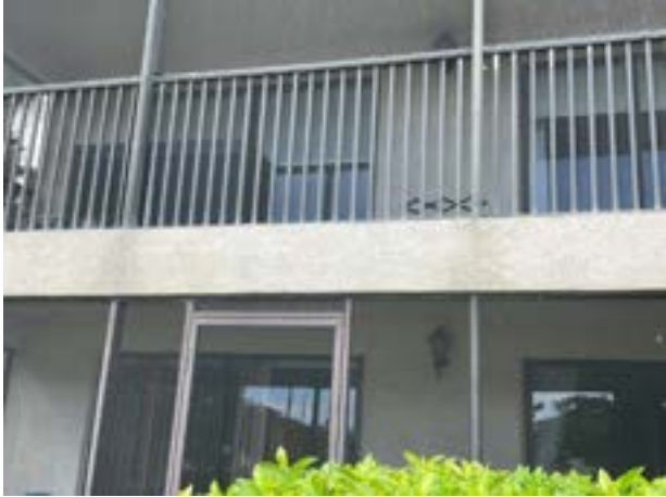
Evidence of moisture
