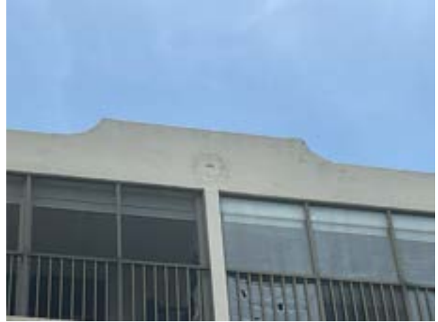
Stucco finish deterioration
