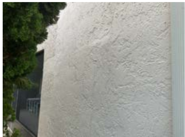
Stair step stucco cracks
