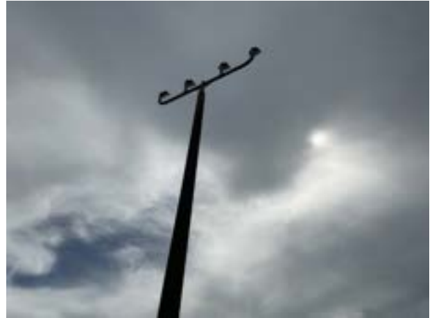
Light pole and fixture
