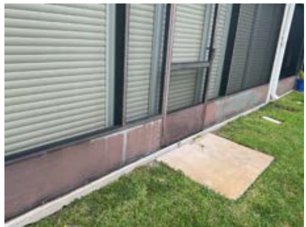
Frame finish deterioration
