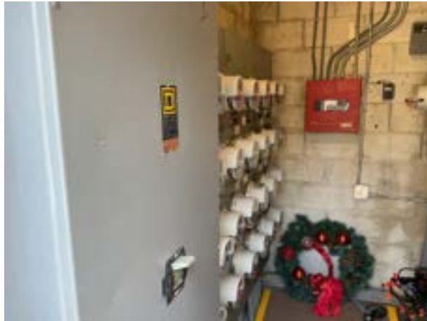
Electrical system components
