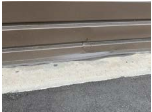
Garage door damage
