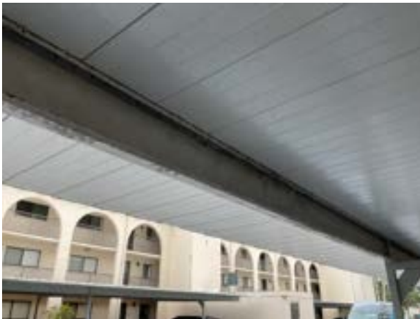
Rusted metal frame
