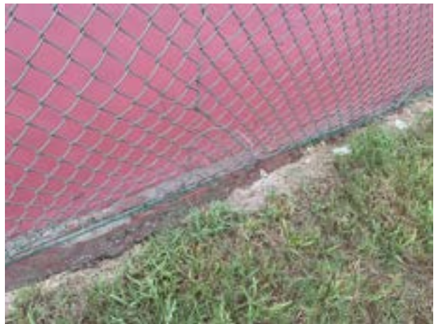
Warped chain link fence
