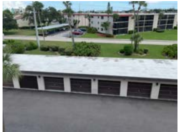
Foam roof with standing water
