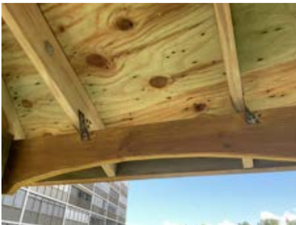
Rusted rafter ties
