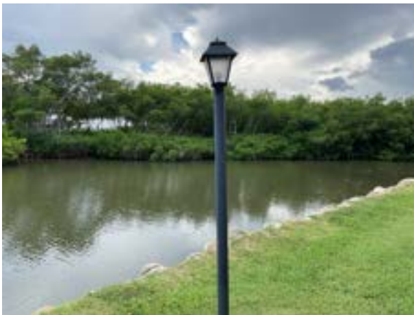
Light pole and fixture
