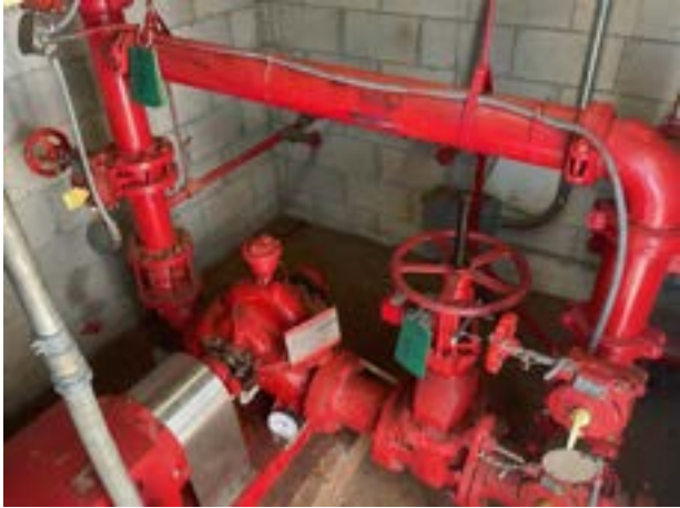
Fire suppression pump
