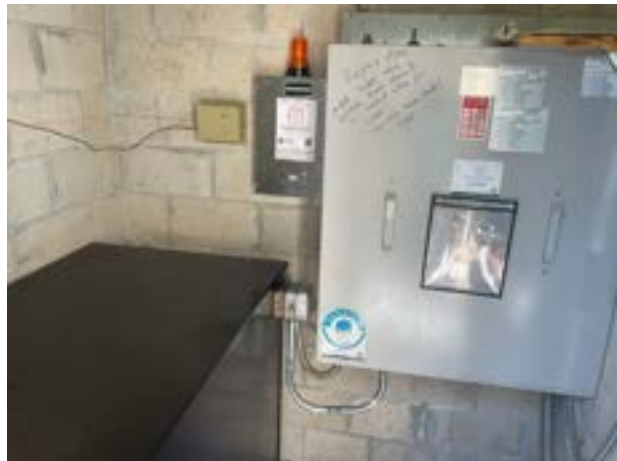
Building 12 elevator equipment
