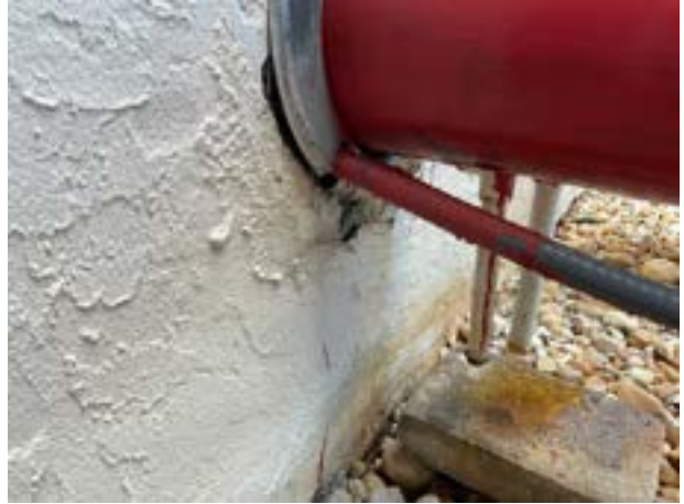
Peeling finish near fire outlet pipe
