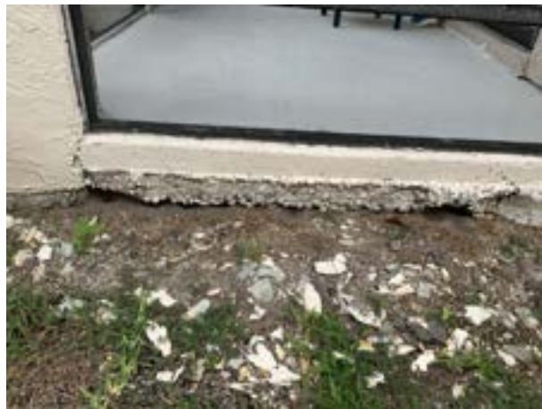
Undermining at on-grade balcony
