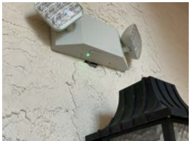
Spall at device connection
