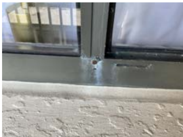
Frame finish deterioration
