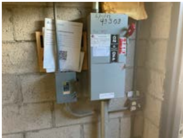
Elevator electrical system components
