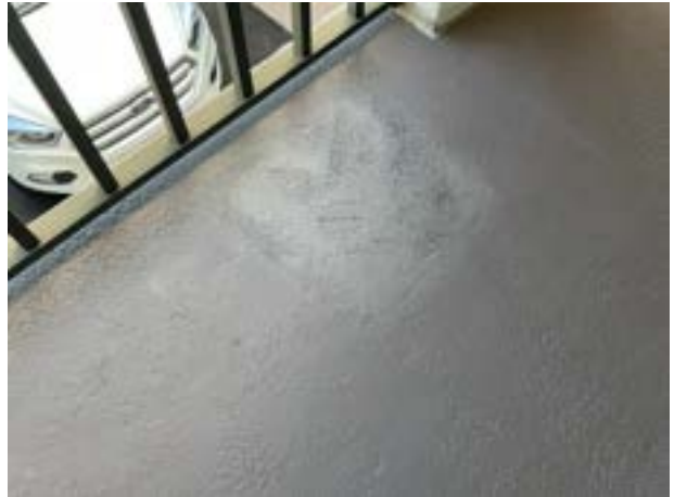
Evidence of previous replacement
