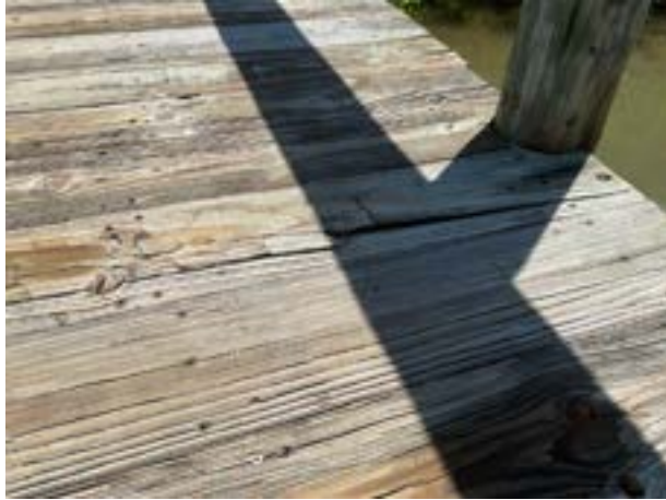
Splintered wood deck
