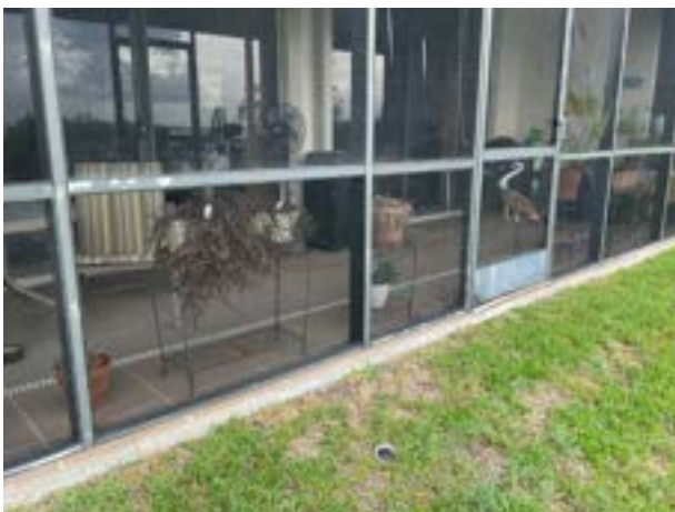
Frame finish deterioration
