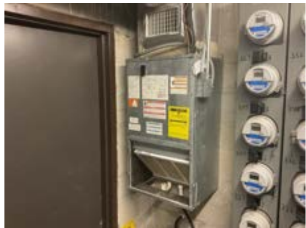
Air handling unit
