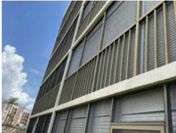
Aluminum railings with finish deterioration
