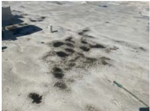
Evidence of standing water
