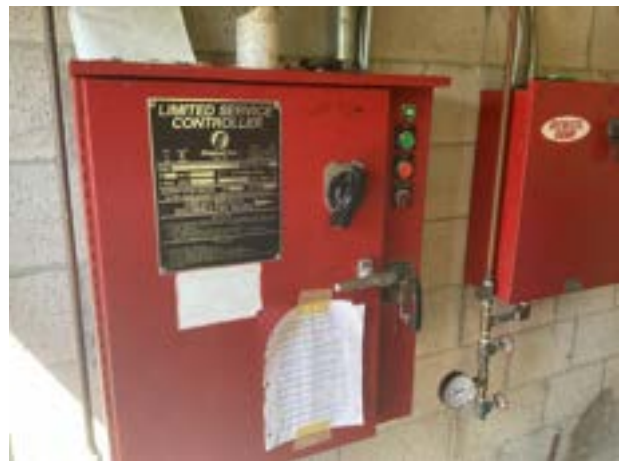
Fire suppression pump control panel
