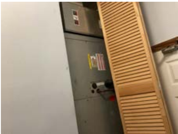
Air handling unit at clubhouse
