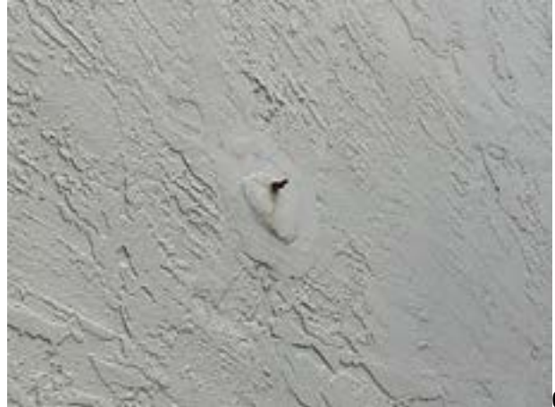
Penetration at stucco
