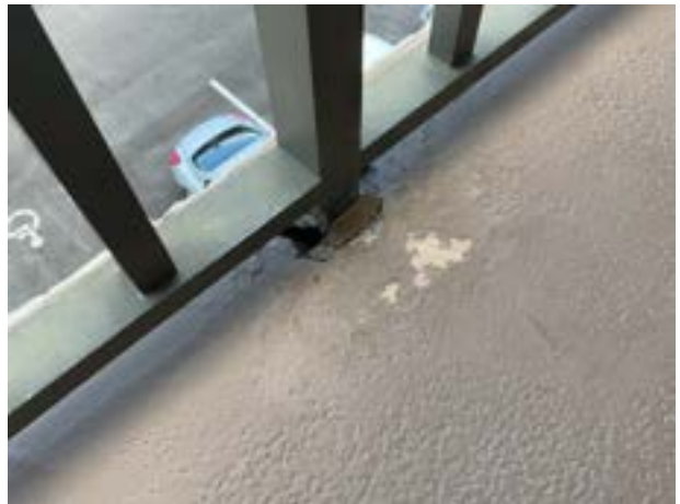
Deterioration at railing breezeway connection
