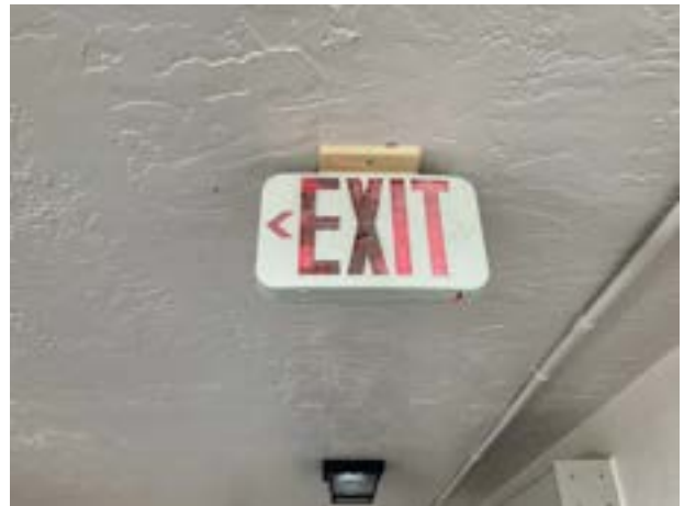
Cracked exit sign
