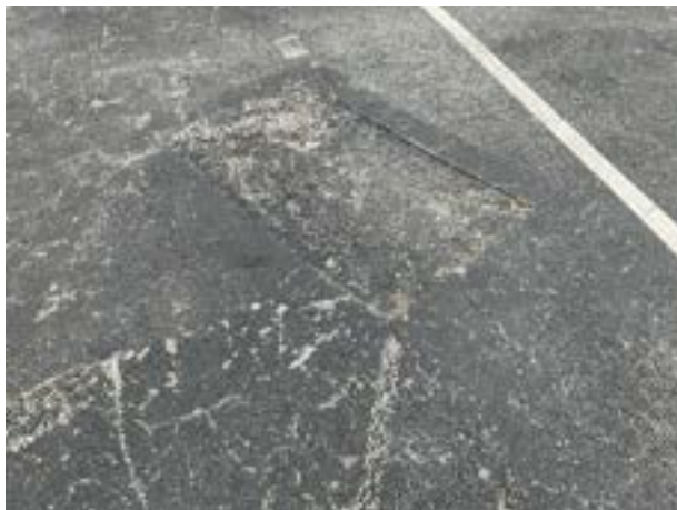
Evidence of previous repairs
