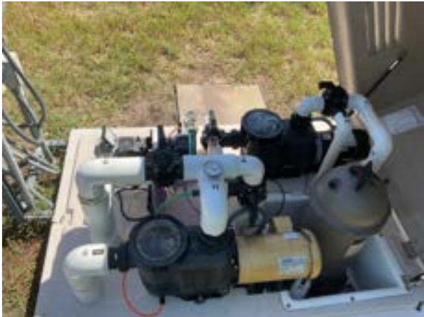
Pool mechanical equipment
