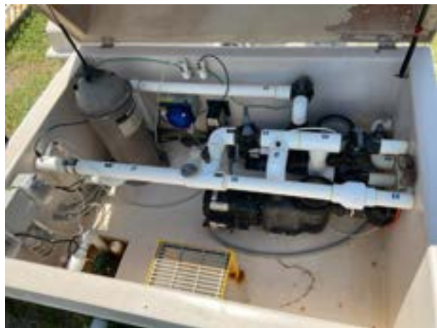
Pool mechanical equipment
