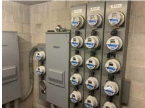
Electrical system components
