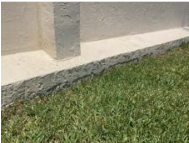
Finish deterioration near grade
