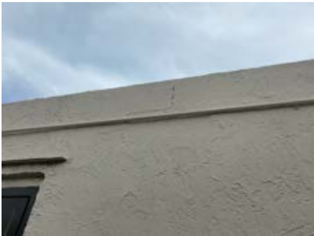
Stair step crack
