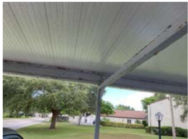
Rusted metal frame
