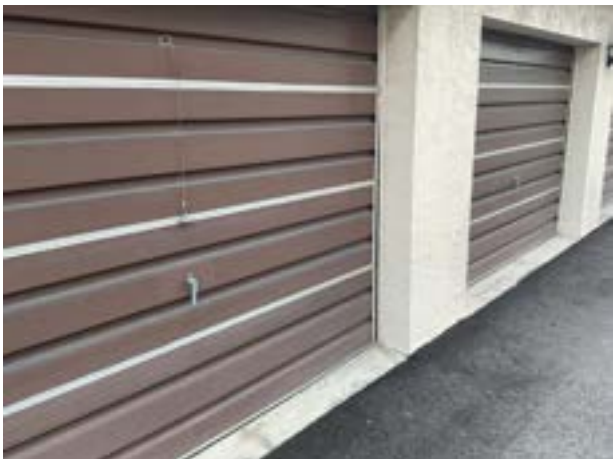
Garage door not on track
