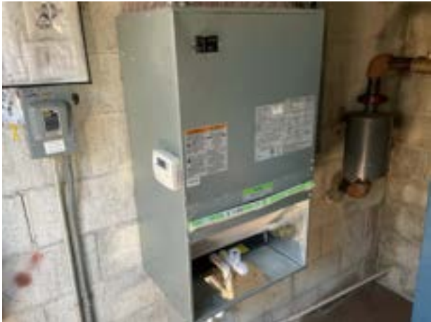
Air handling unit
