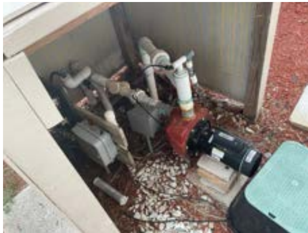
Irrigation pump and controller
