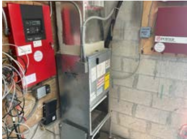
Air handling unit
