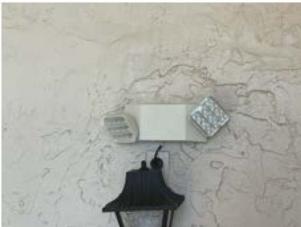
Emergency light fixture
