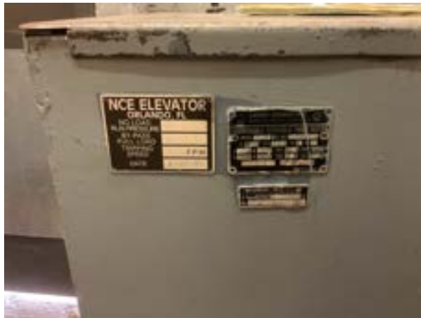
Building 11 elevator equipment information
