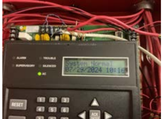
Operational control panel
