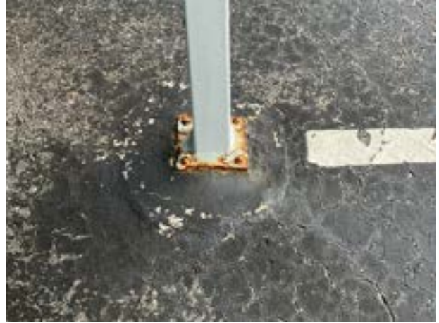
Rusted metal frame
