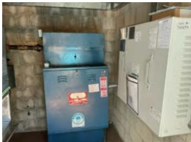
Building 2 elevator equipment
