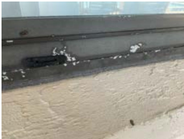
Sealant deterioration at clubhouse windows
