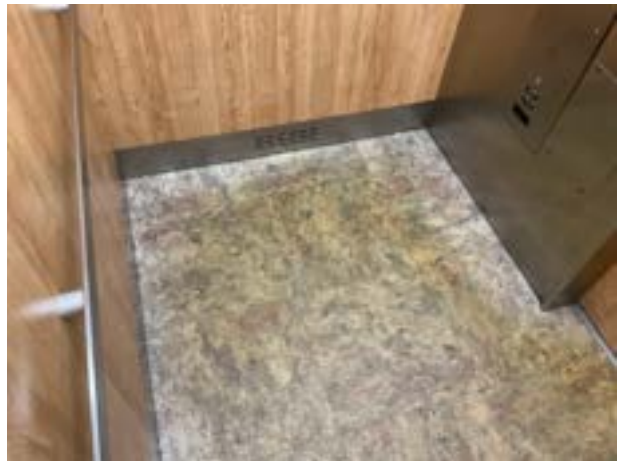
Tile floor coverings with faded finish
