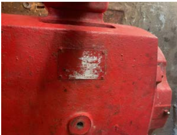
Fire suppression pump tag
