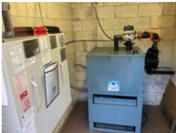
Building 1 elevator equipment
