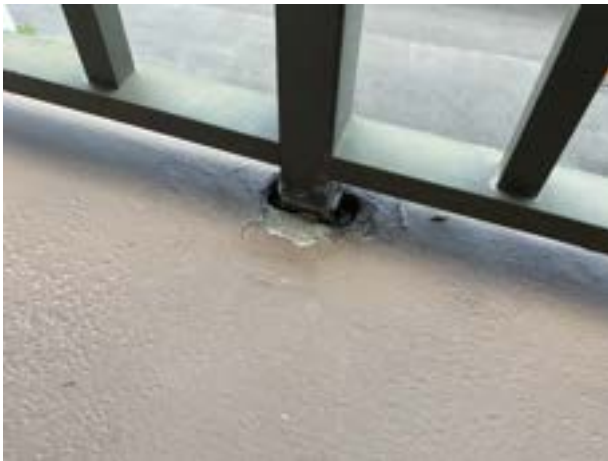
Deterioration at railing breezeway connection
