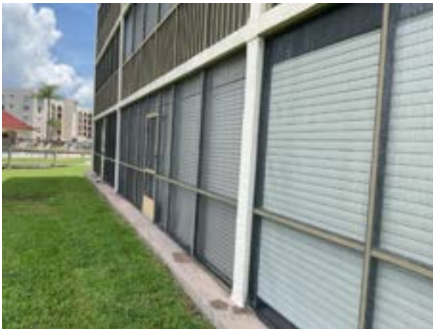
Balcony screens with frame finish deterioration
