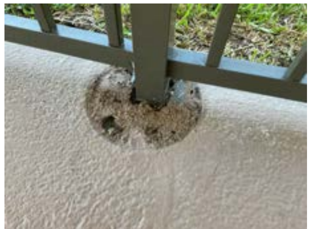
Deterioration at fence post connection
