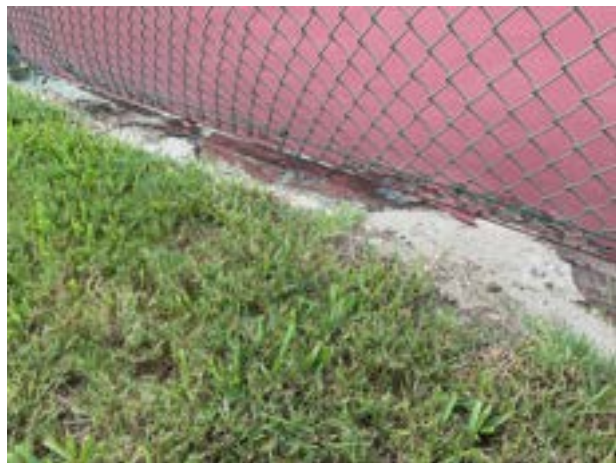
Surface deterioration at edge
