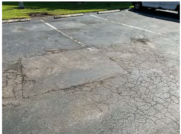
Asphalt pavement cracks
