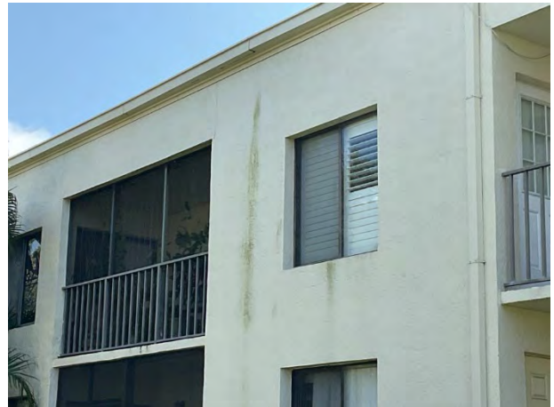
Stucco finish stains
