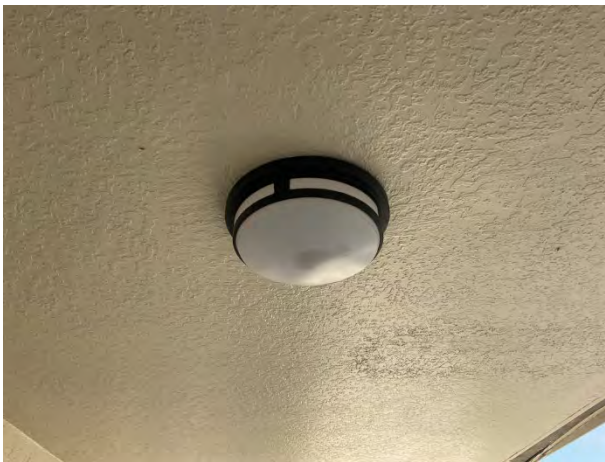
Breezeway exterior light fixture
