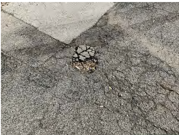
Asphalt pavement pothole
