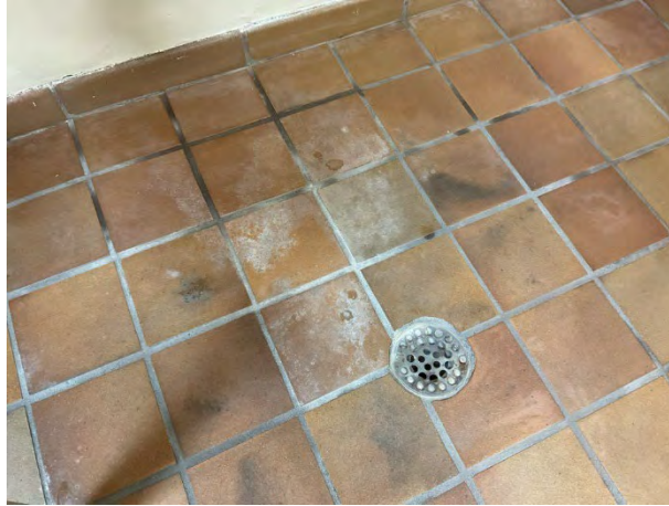
Tile finish deterioration
