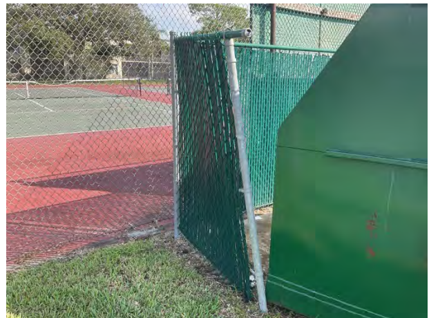
Fence leaning section
