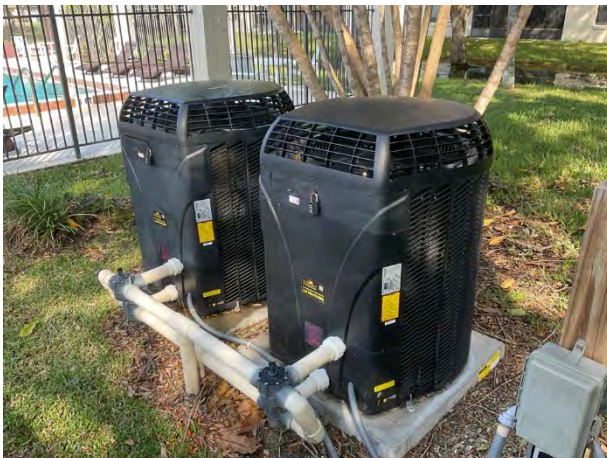
Pool mechanical equipment
