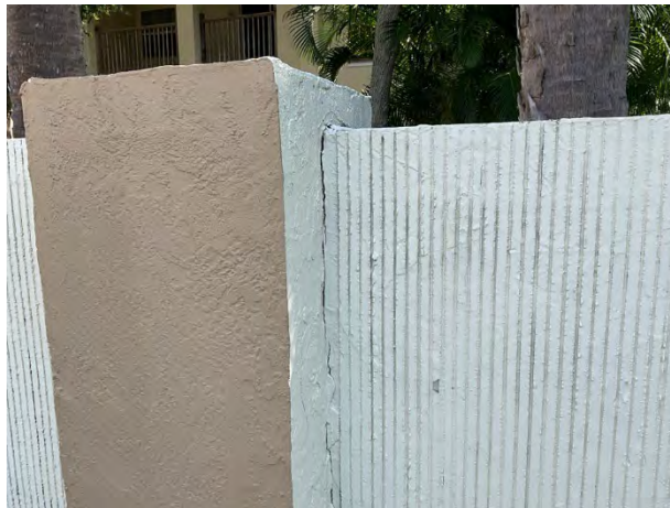
Wall stucco cracks
