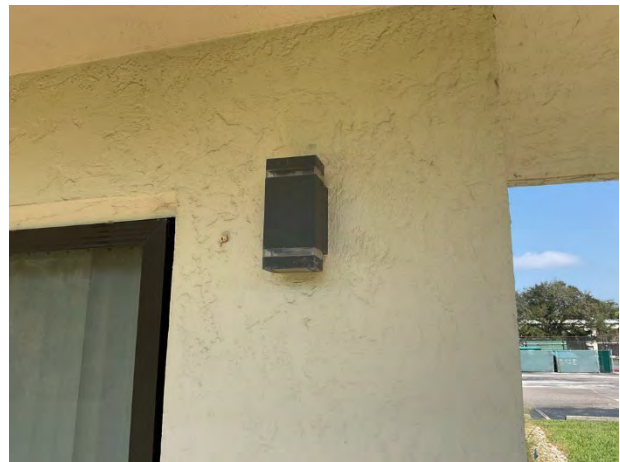
Balcony exterior light fixture
