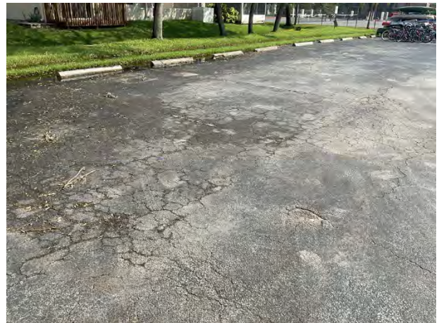
Asphalt pavement cracks
