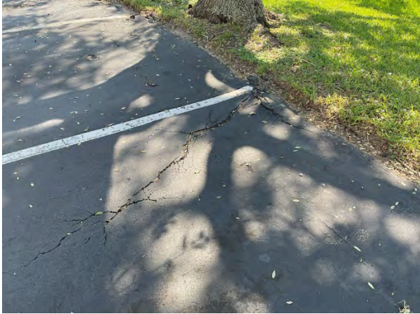
Asphalt pavement cracks
