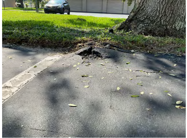
Asphalt pavement upheaval
