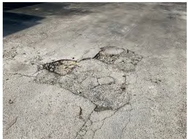
Asphalt pavement cracks and potholes
