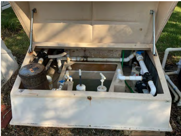
Pool mechanical equipment
