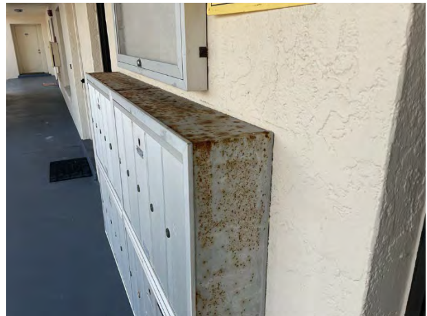
Mailbox station rust
