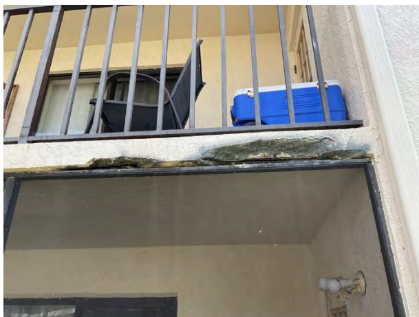
Balcony edge deterioration
