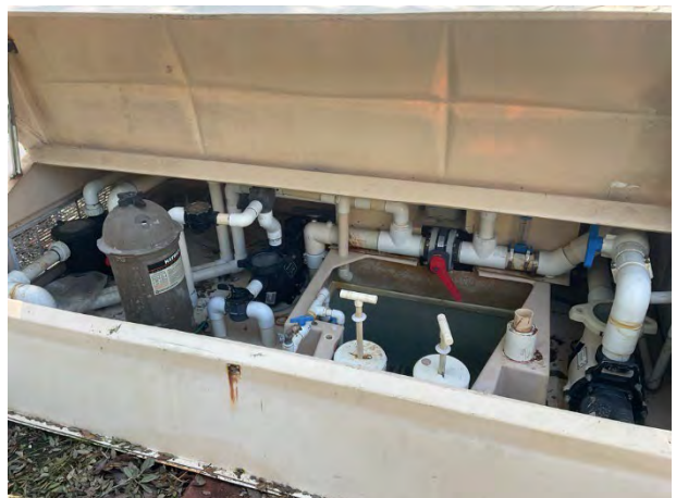
Pool mechanical equipment
