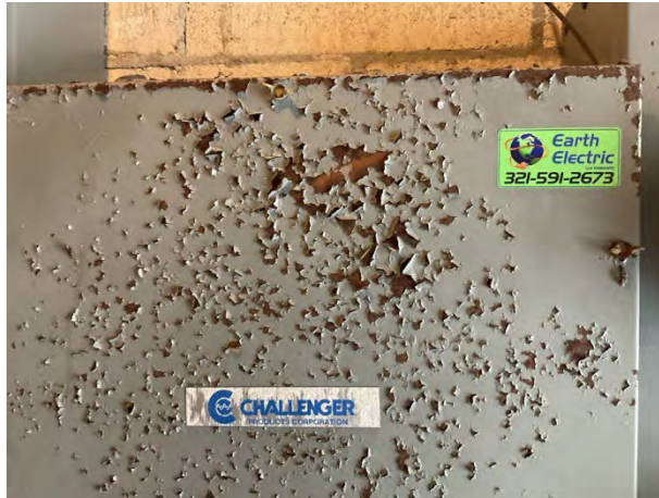
Electrical system rust and peeling paint
