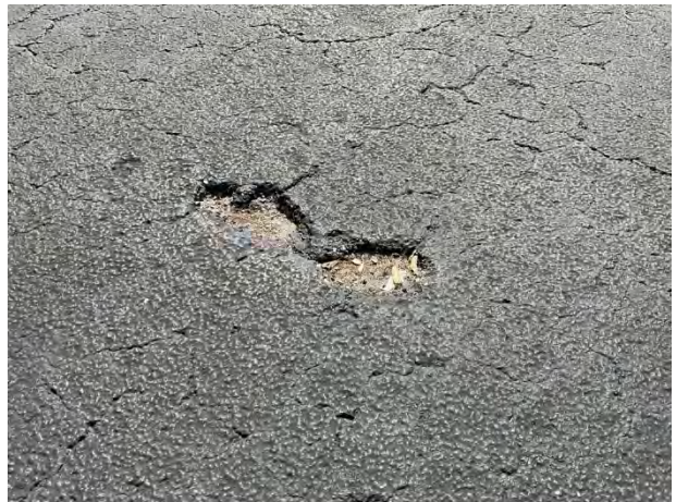
Asphalt pavement spall
