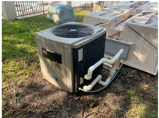
Pool mechanical equipment
