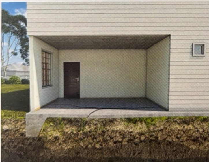
BEFORE: Slab settlement due to soil settlement
