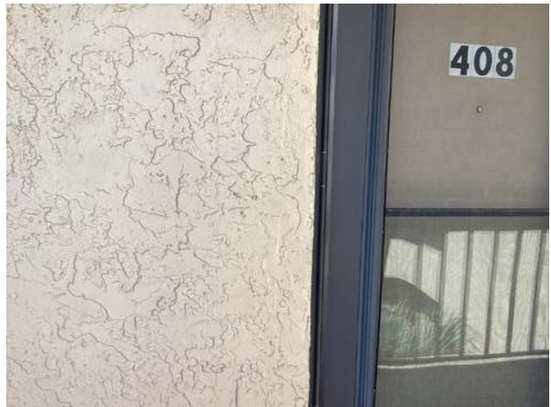
Stucco damage at unit 408 entrance
