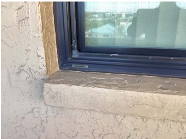
Sealant deterioration at unit 406 front window
