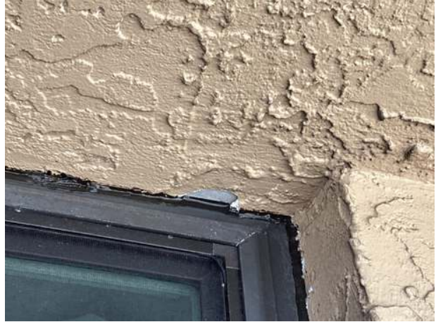
Finish deterioration at underside of third floor breezeway at unit 212 front window
