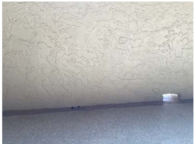
Stucco cracks at unit 305
