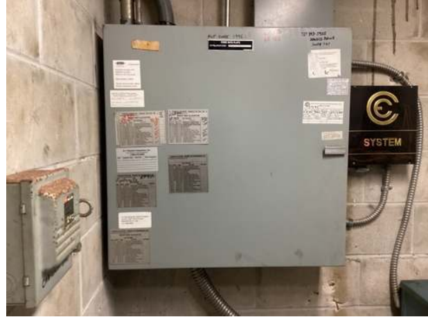
Hydraulic elevator controls
