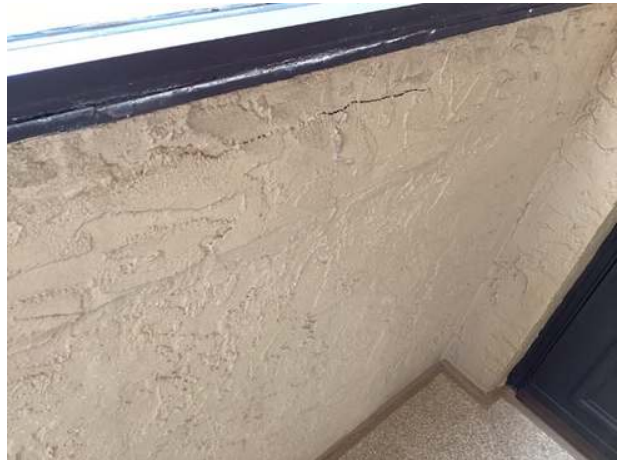
Stucco cracks at second floor breezeway
