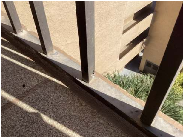
Finish deterioration at fifth floor breezeway
