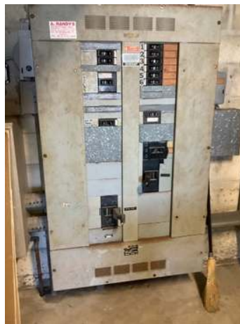
Switchgear for common areas
