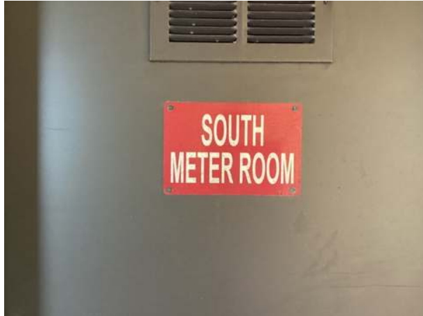
Electrical room label
