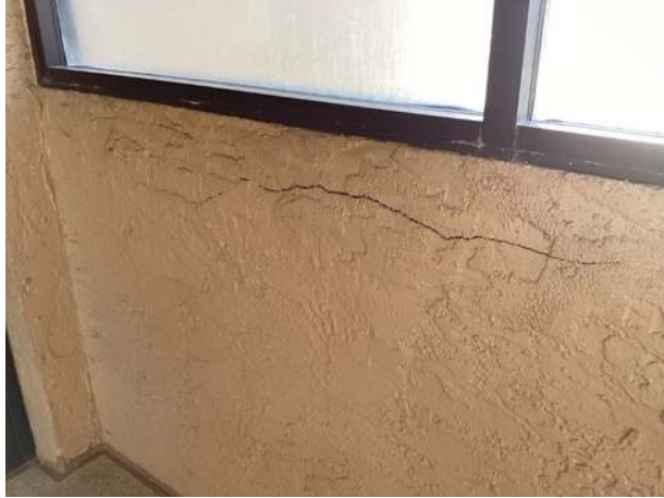
Stucco cracks at unit 507 entrance
