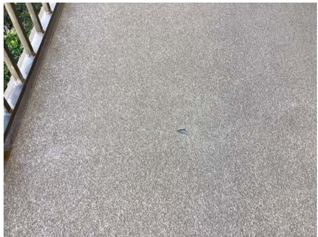
Isolated cracks and coating deterioration at unit 102 entrance
