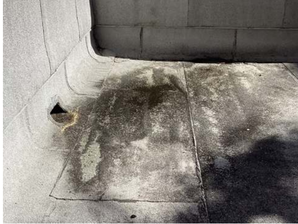
Standing water at the lobby roof
