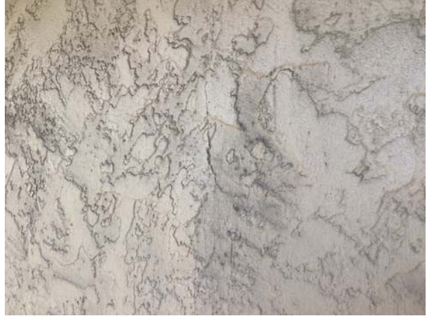
Stucco cracks and damage at 5th floor breezeway across from north tower trash room
