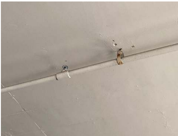
Rust at pipes
