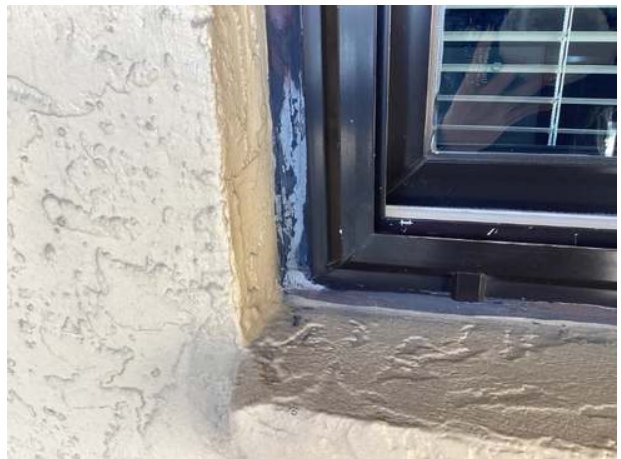
Sealant deterioration at unit 505 front window
