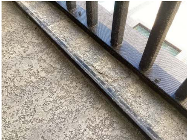
Coating delamination at unit 204
