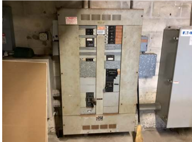
Electrical system main panel
