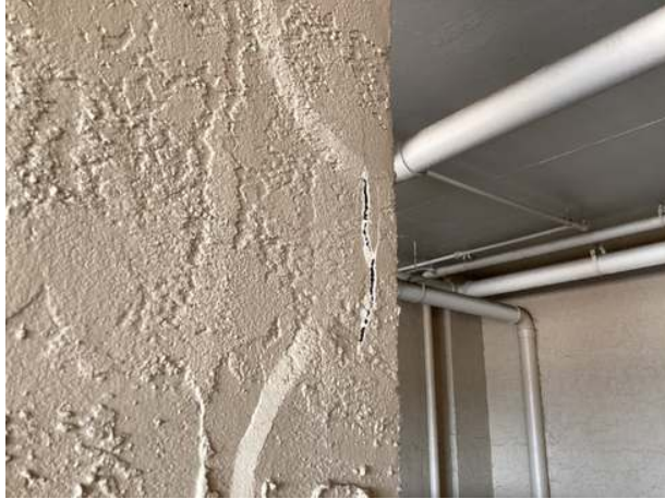
Stucco crack at garage
