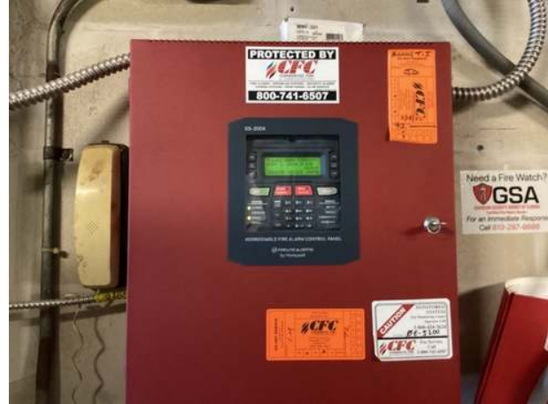
Control panel reports trouble in the system
