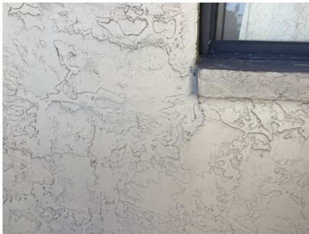
Stucco cracks at unit 213 front window
