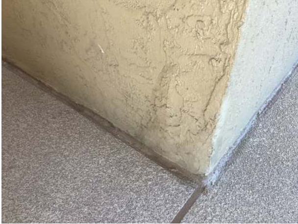
Stucco deterioration outside fourth floor north tower trash room
