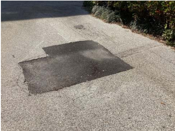
Pavement cracks, patches and settlement
