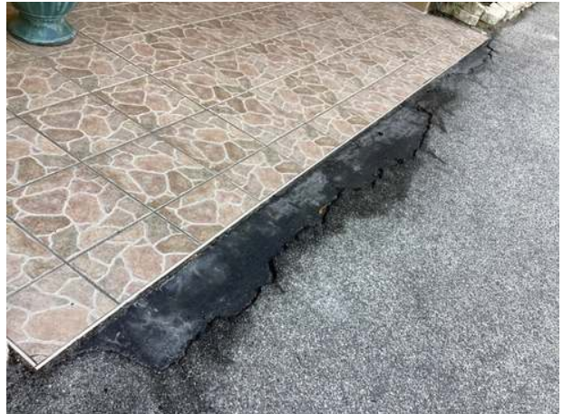
Pavement edge deterioration
