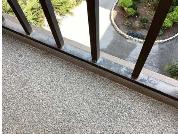
Railing finish deterioration at fifth floor
