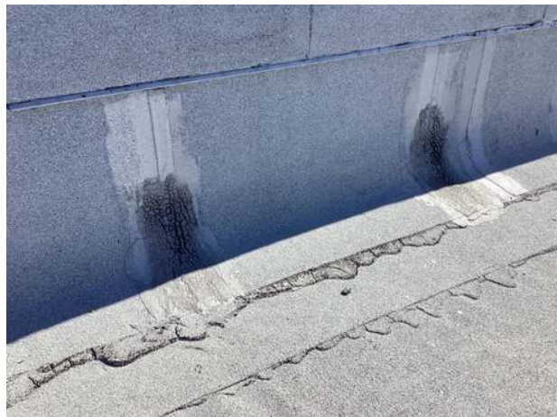
Cracks in sealant throughout
