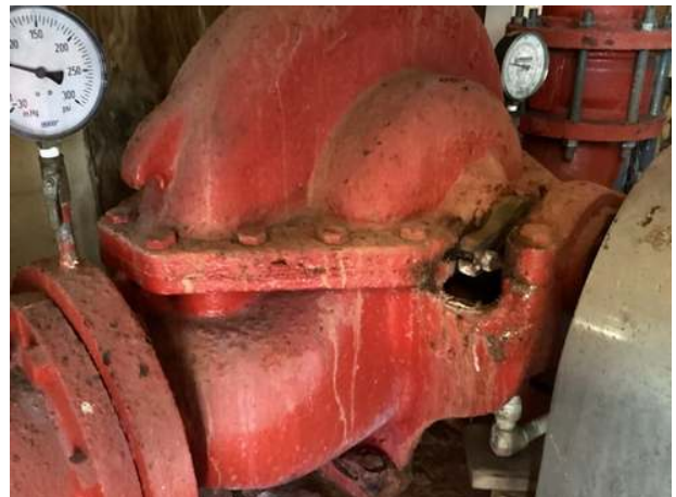
Fire suppression pump
