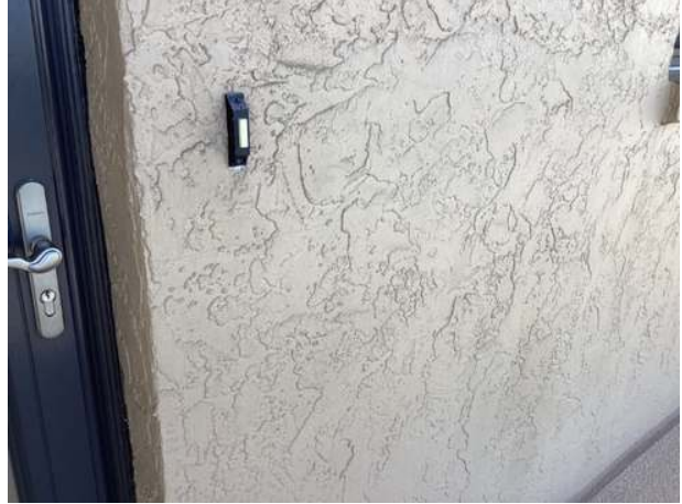
Stucco cracks at unit 508 front entrance
