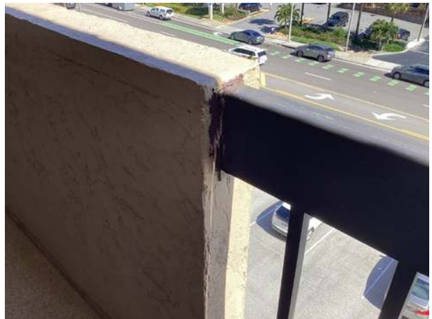
Loose connection outside unit 410
