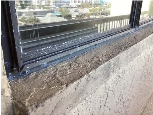
Sealant deterioration at unit 303 front window
