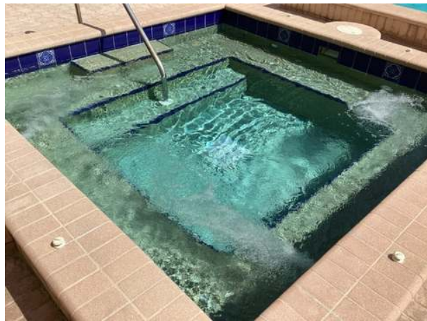
Spa overview with stained plaster
