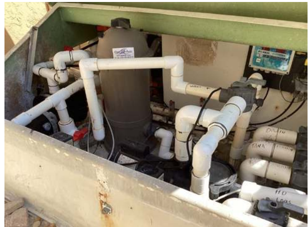
Pool mechanical equipment
