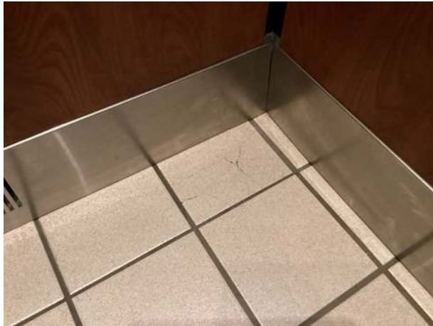
Cracked elevator cab tile
