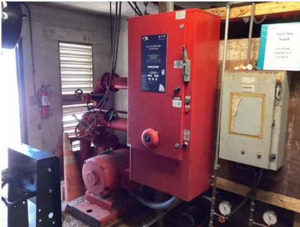
Fire suppression pump and controls
