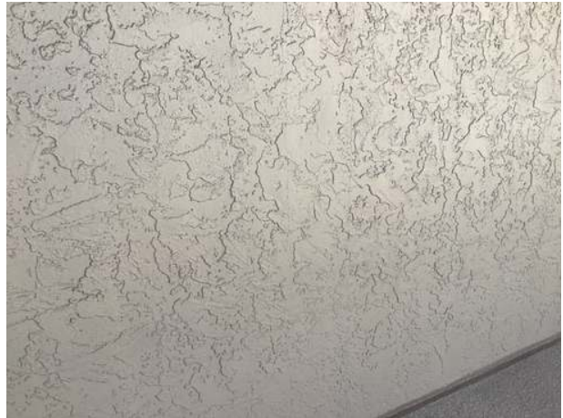
Stucco cracks in between units 506 and 507
