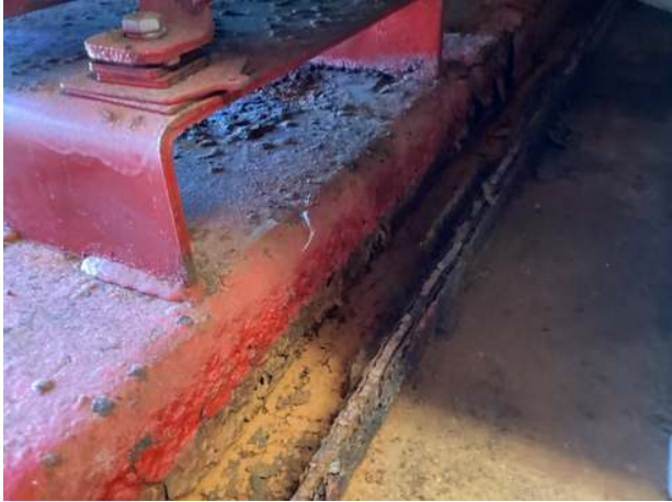
Rust at base
