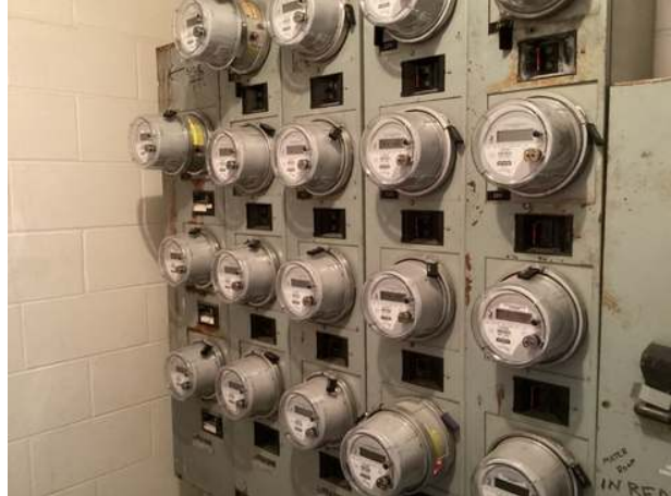
South tower meters rust evident
