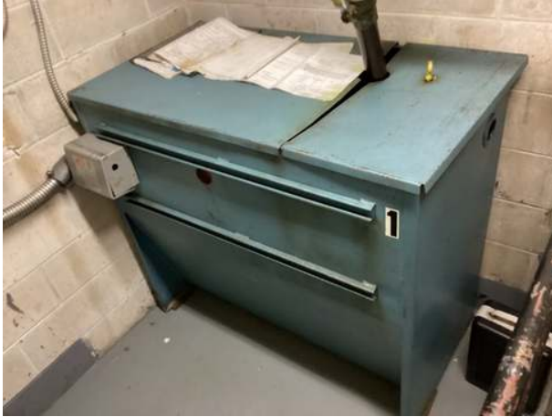
Hydraulic elevator equipment
