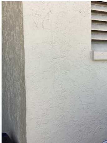
Stucco cracks near generator room entrance
