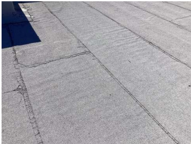
Wrinkles evident at the south elevation of the south tower
