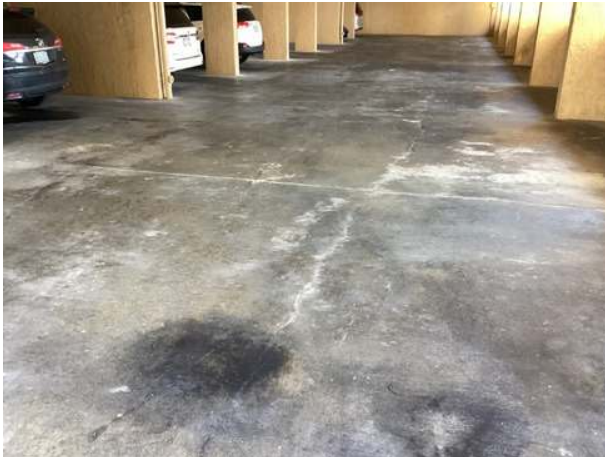
On-grade concrete garage floor with cracks
