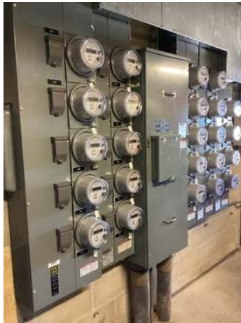
Electrical meters for building b center building recent replacements
