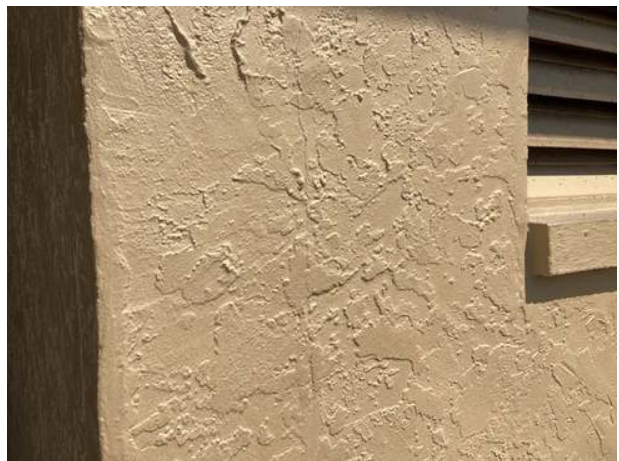
Stucco crack at fire alarm room
