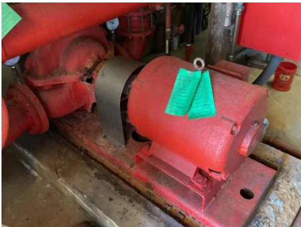
Fire suppression pump
