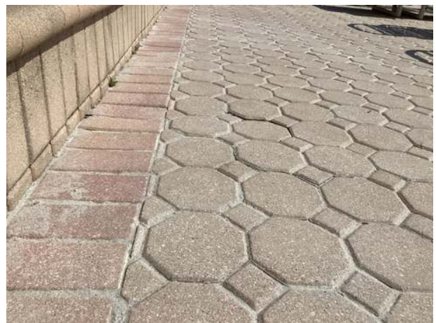
Minor paver settlement
