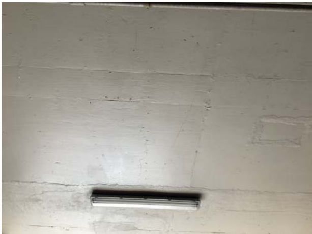
Isolated cracks at underside of the north tower first floor at the south elevation
