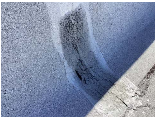
Membrane tear at south tower west parapet wall
