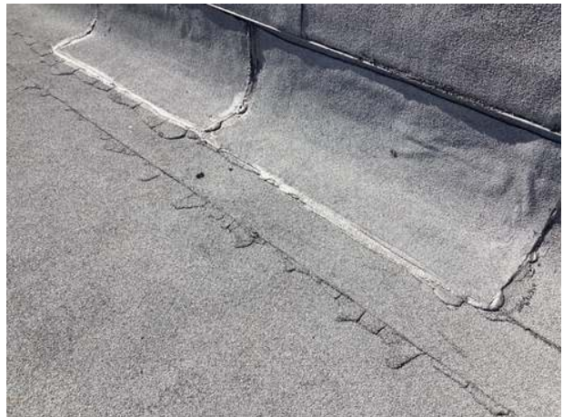
Recent repairs evident at the west elevation parapet of the north tower
