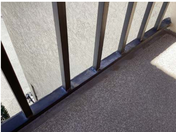
Railing finish fade at second floor north tower breezeway
