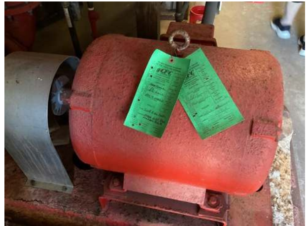
Fire suppression pump motor
