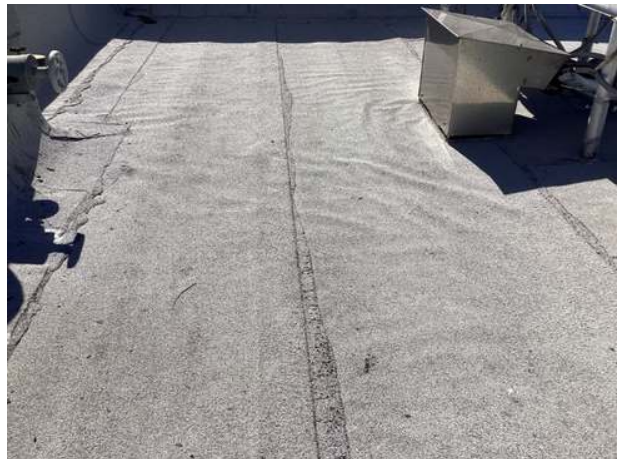
Wrinkles evident at the south west corner of the south tower roof
