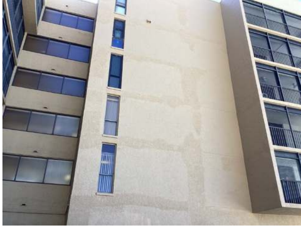
Inconsistent finishes Evident at the north elevation of the center tower
