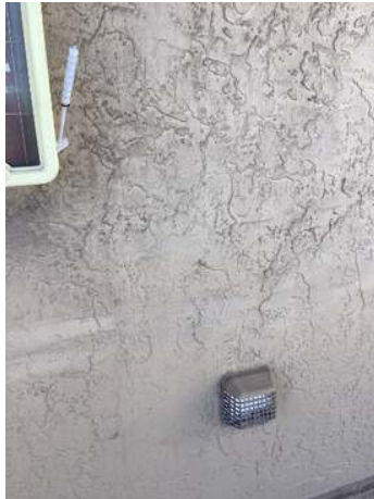
Stucco cracks in between units 502 and 503
