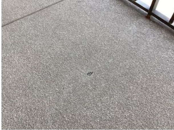
Coating crack and damage at first floor
