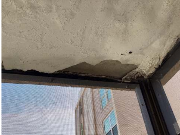
Ceiling damage at common balcony
