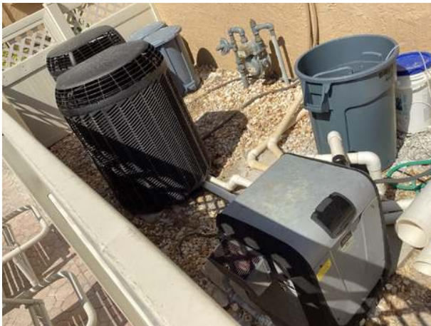
Pool and spa heaters
