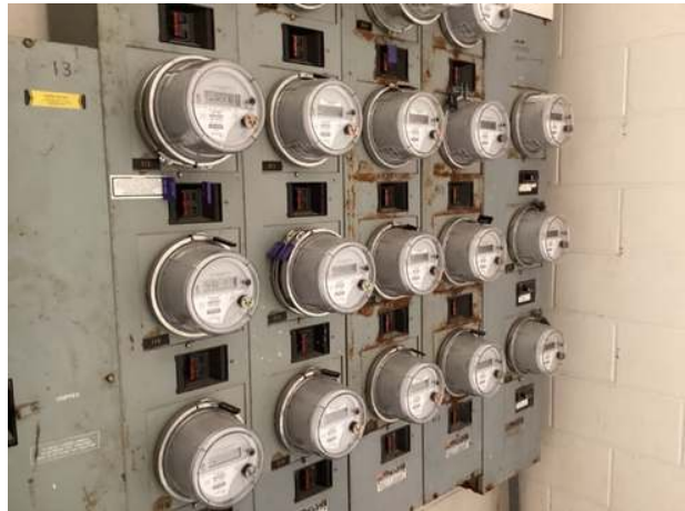
Electrical meters for north tier rust evident
