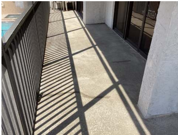
Balcony overview with cracks
