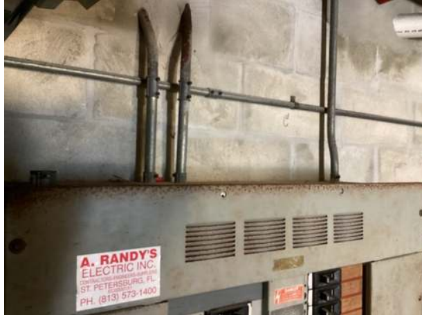
Minor rust evident at common area switchgear
