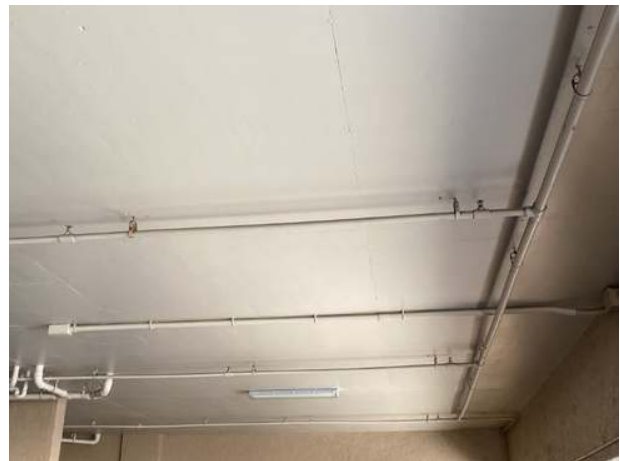
Fire suppression system
