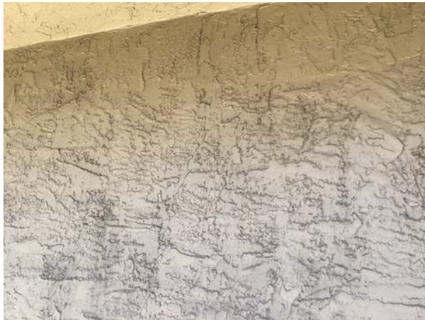
Stucco cracks at fourth floor outside the north tower trash room
