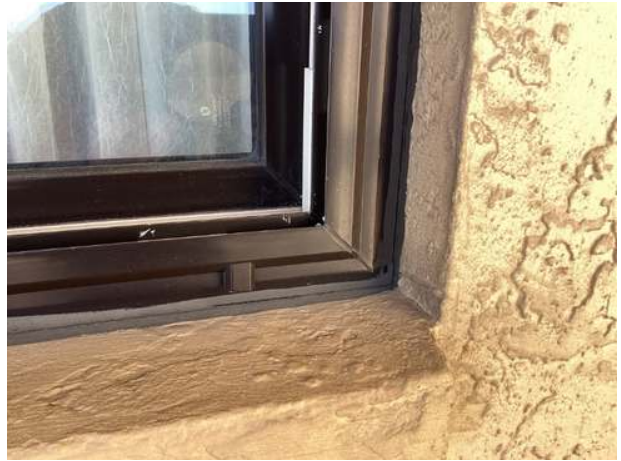
Sealant deterioration at unit 404 front window
