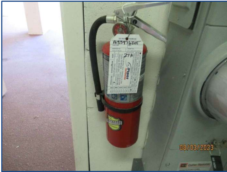
Photograph No. 27: Fire extinguisher
