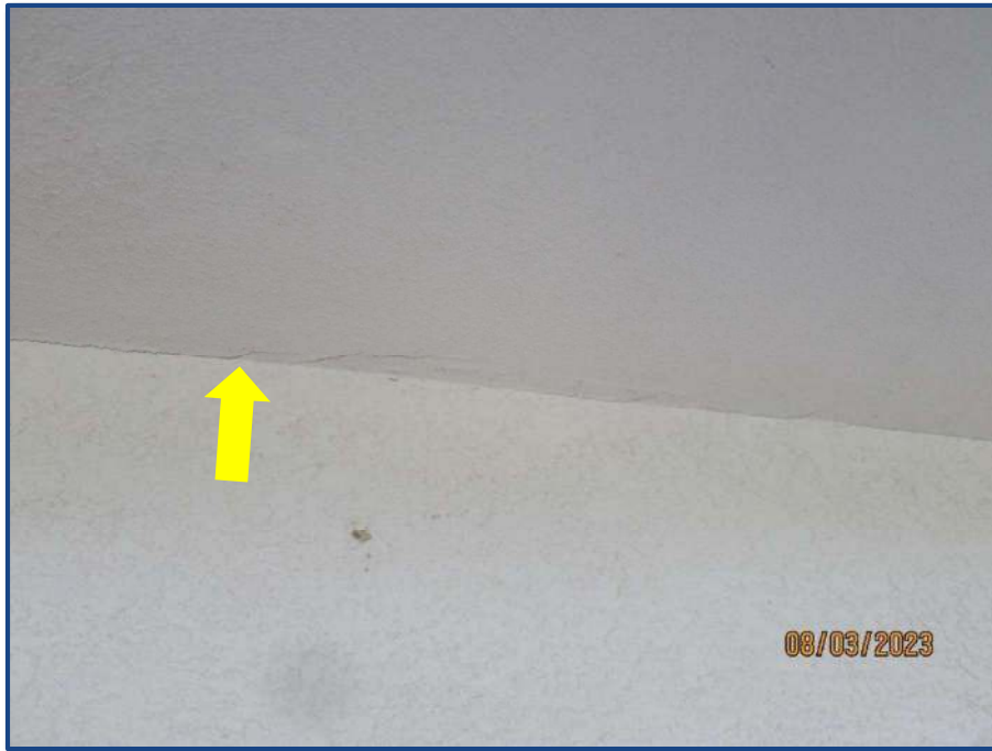
Photograph No. 15: View of crack in the exterior ceiling finish located in the balcony of Unit 6506.
