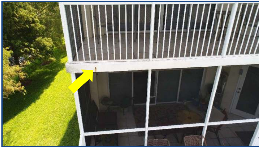
Photograph No. 7: View of surface corrosion and rust staining along the balcony edge located at the 2nd floor balcony.
