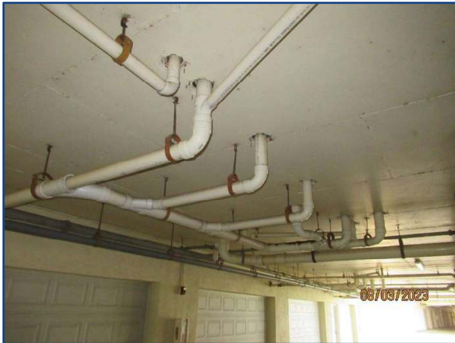
Photograph No. 34: General view of the plumbing located at the garage floor.
