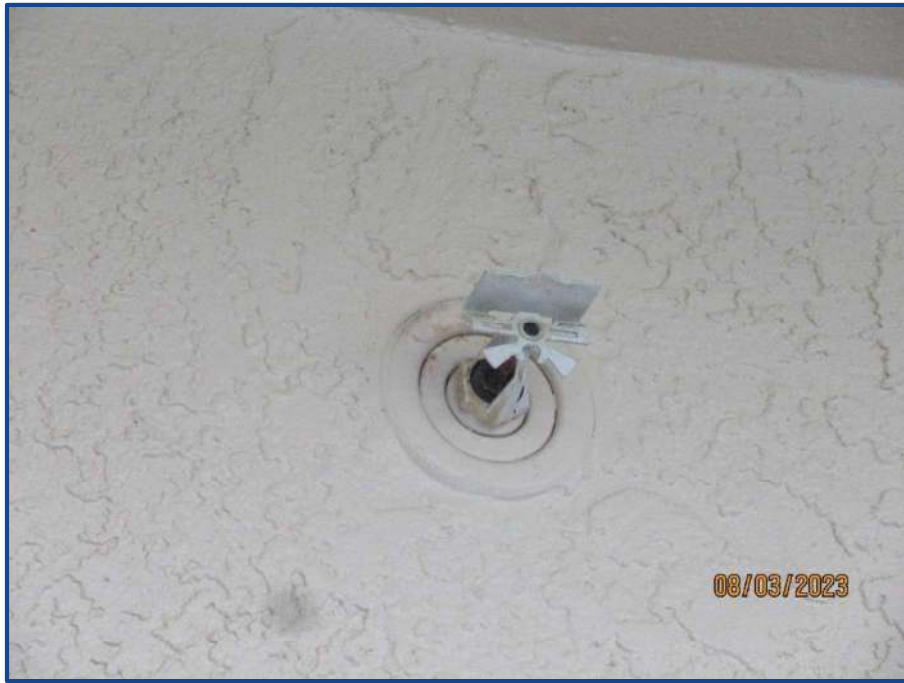
Photograph No. 25: Fire sprinkler head.
