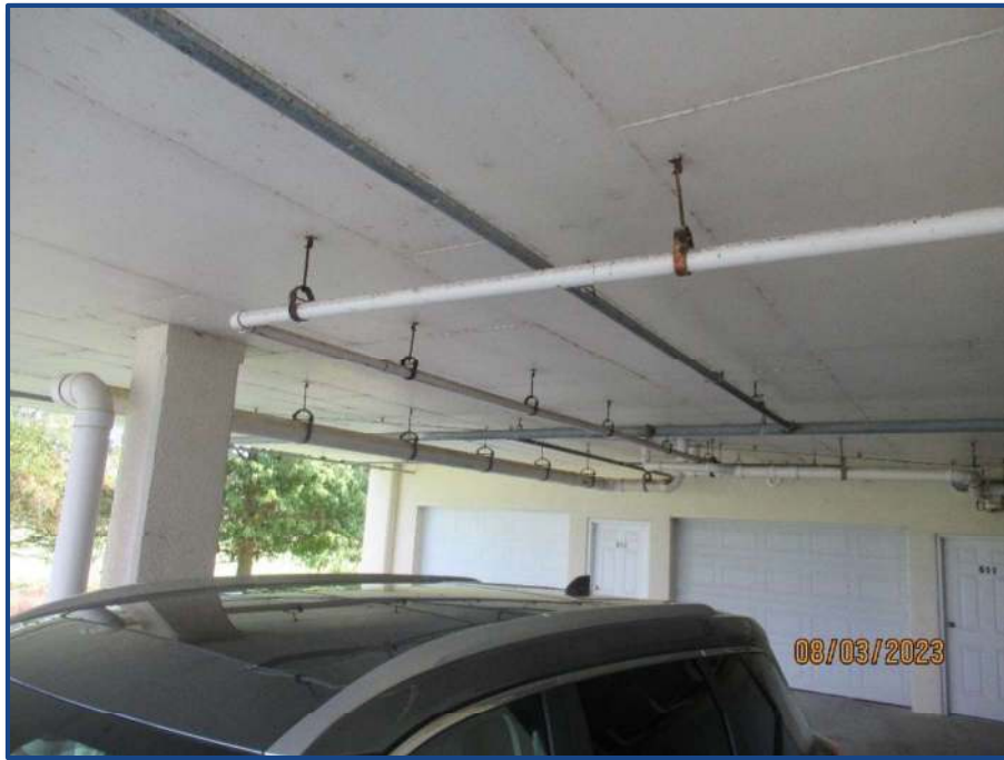
Photograph No. 31: General view of the plumbing located at the garage floor.
