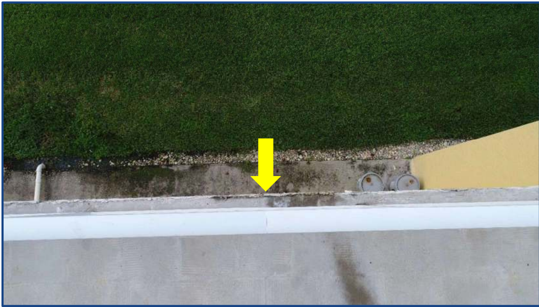
Photograph No. 9: View of stucco damage and separation along the 1st floor balcony slab edge.
