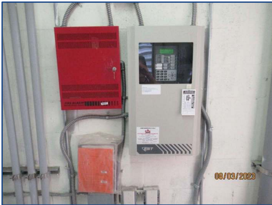
Photograph No. 26: Fire alarm system.
