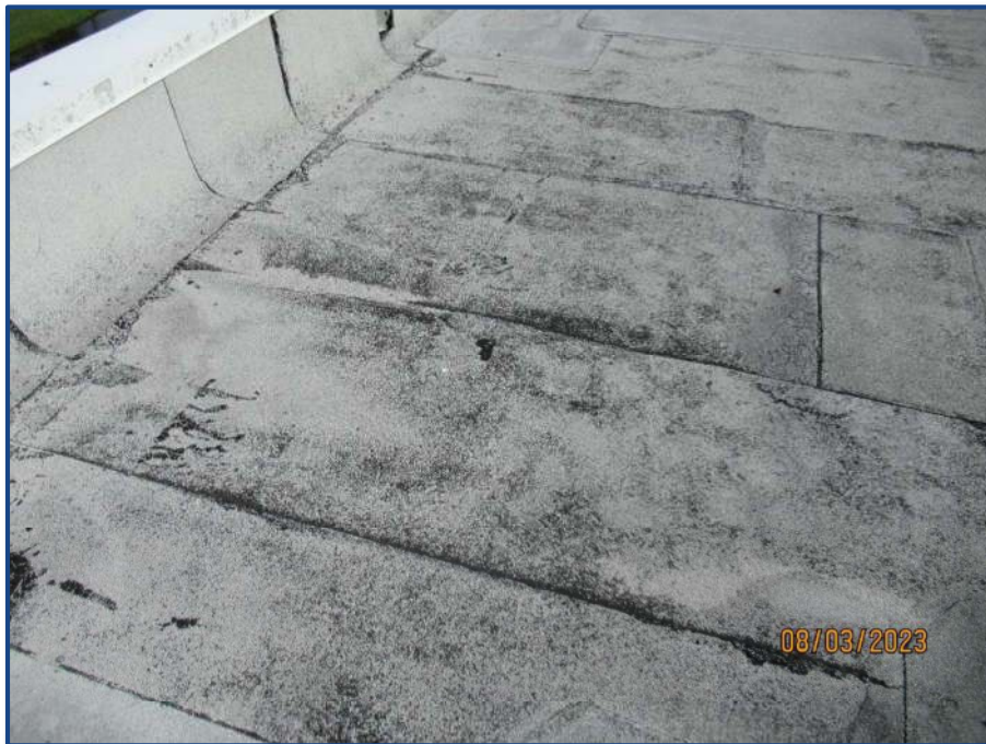
Photograph No. 18: View of granular loss and significant deterioration in the roof membrane.
