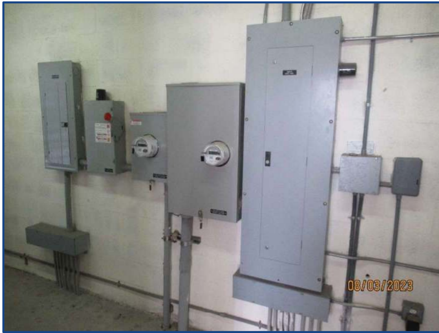
Photograph No. 35: Electrical panels, meters, and conduits.
