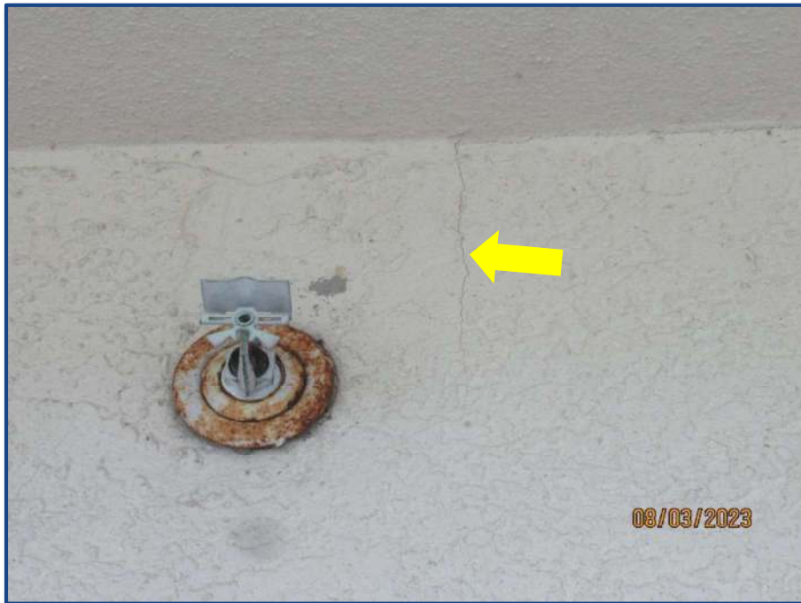
Photograph No. 14: View of crack in the exterior wall stucco finish located in the balcony of Unit 6506.
