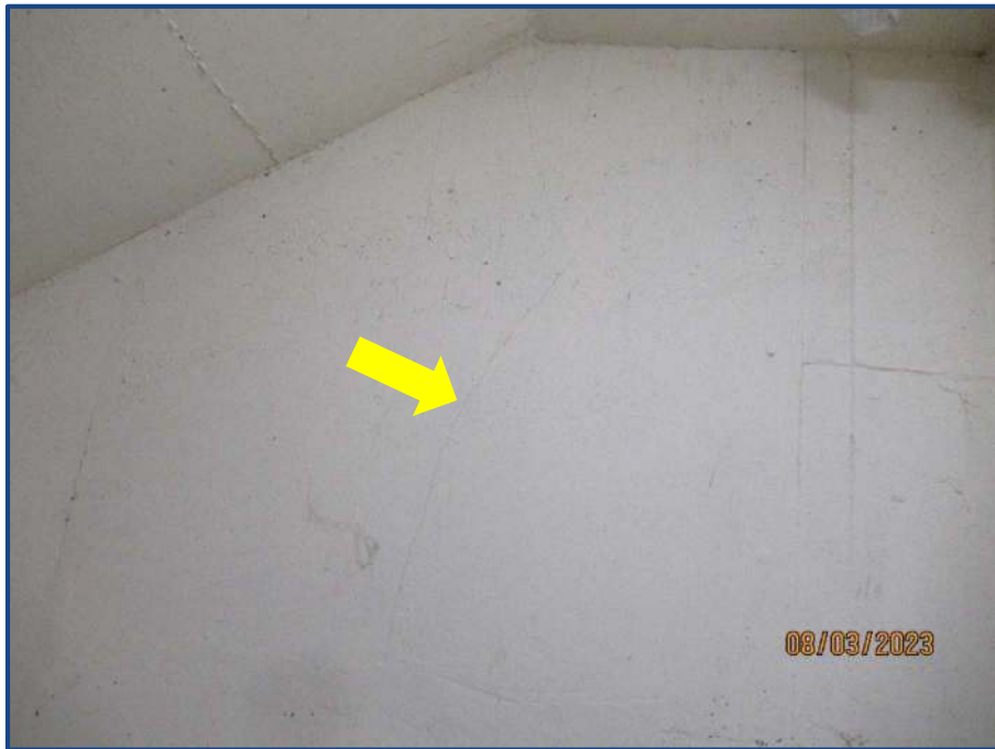
Photograph No. 24: View of crack in the interior wall of Stair 1 Floor 2.
