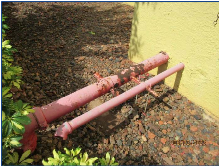
Photograph No. 42: Corroded fire riser pipe.
