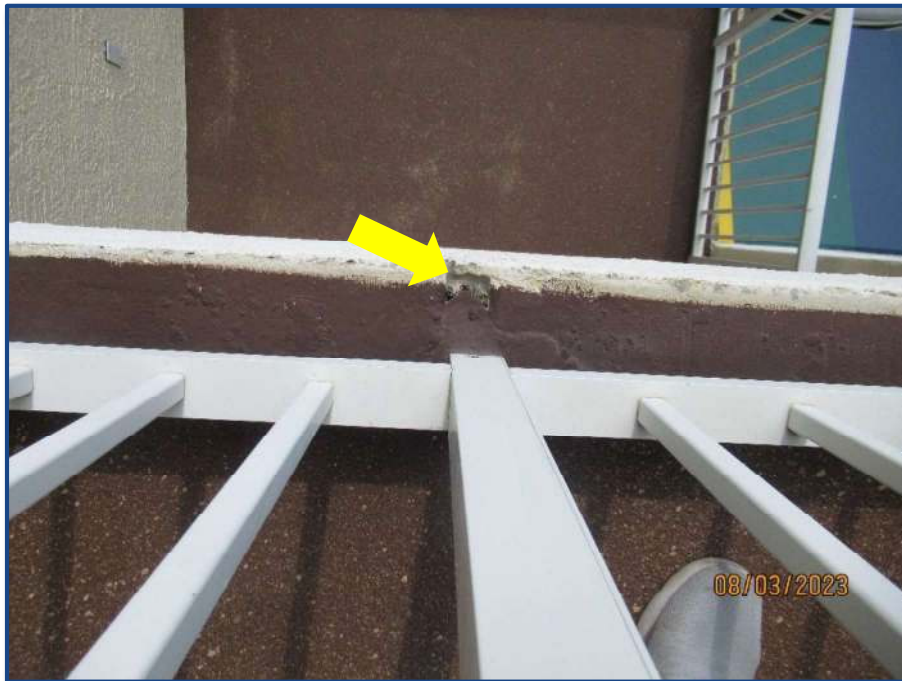
Photograph No. 22: View of void at the exterior walkway railing post located on the 3rd floor.
