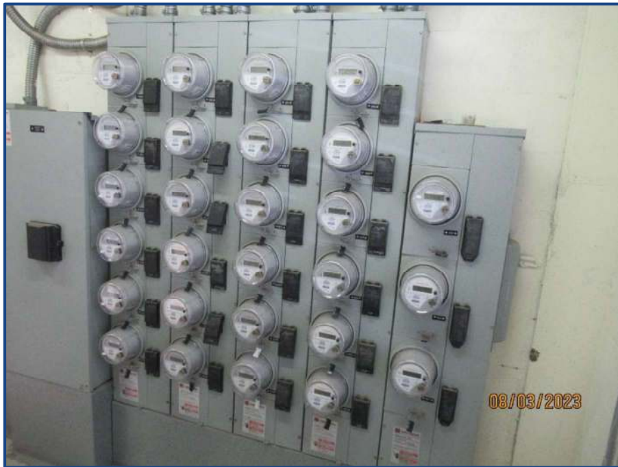
Photograph No. 36: Electrical meters.
