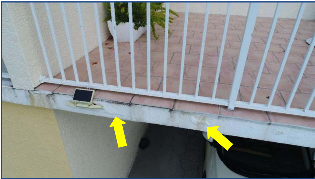
Photograph No. 10: View of bubbling in the exterior stucco finishes located along the exterior balcony edge.
