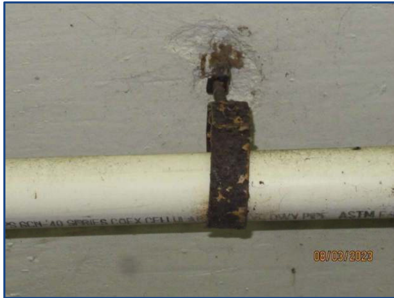
Photograph No. 33: View of corroded plumbing hangers located in the garage level.
