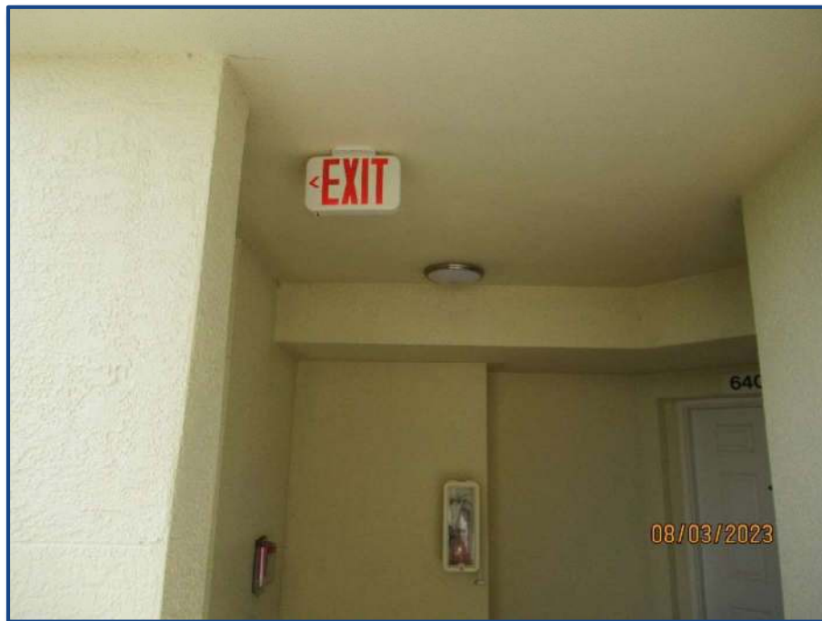
Photograph No. 30: View of fire alarm pull station, fire extinguisher, and emergency exit sign.
