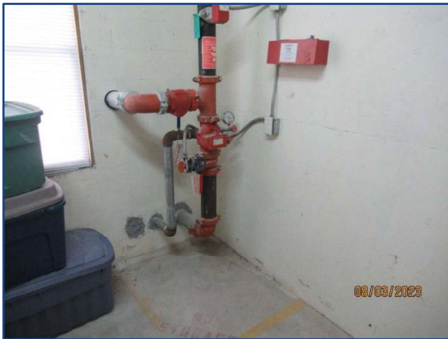
Photograph No. 28: Fire riser system.
