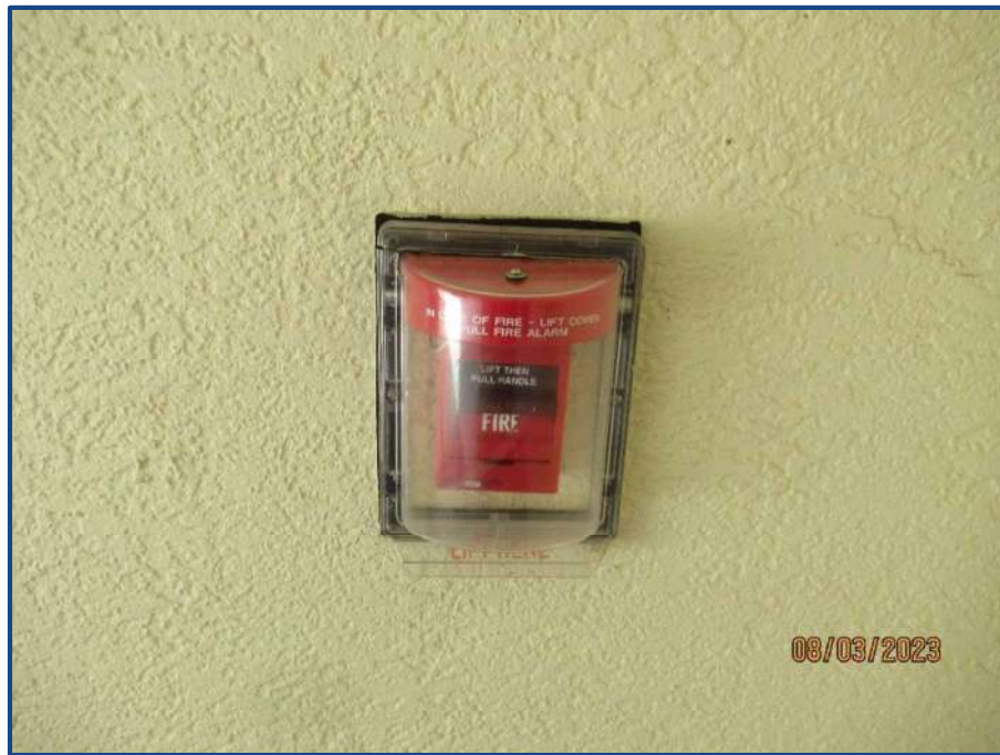
Photograph No. 29: Fire alarm pull station.
