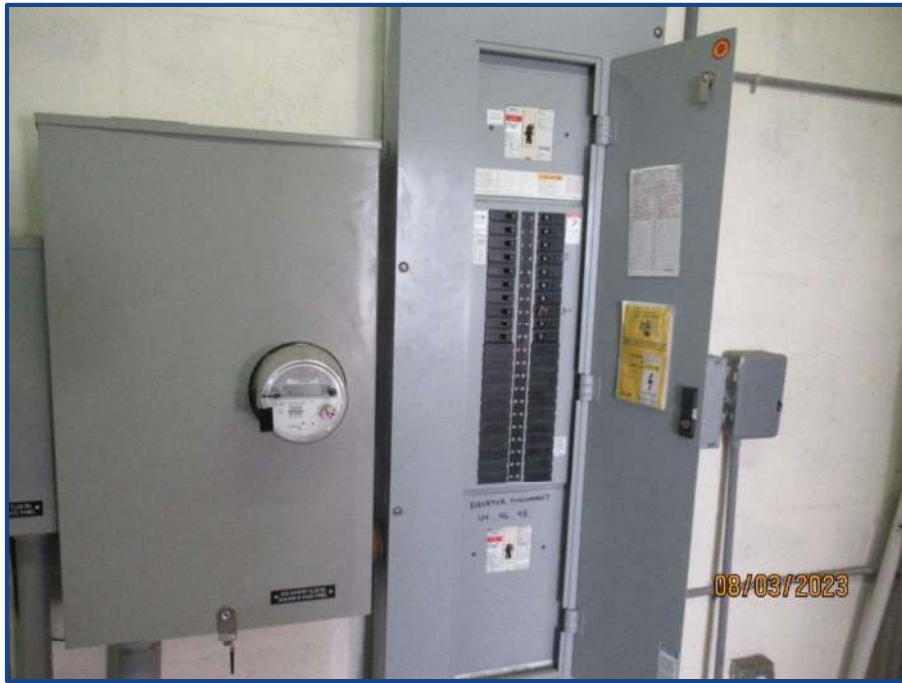
Photograph No. 37: Electrical meter and panel.
