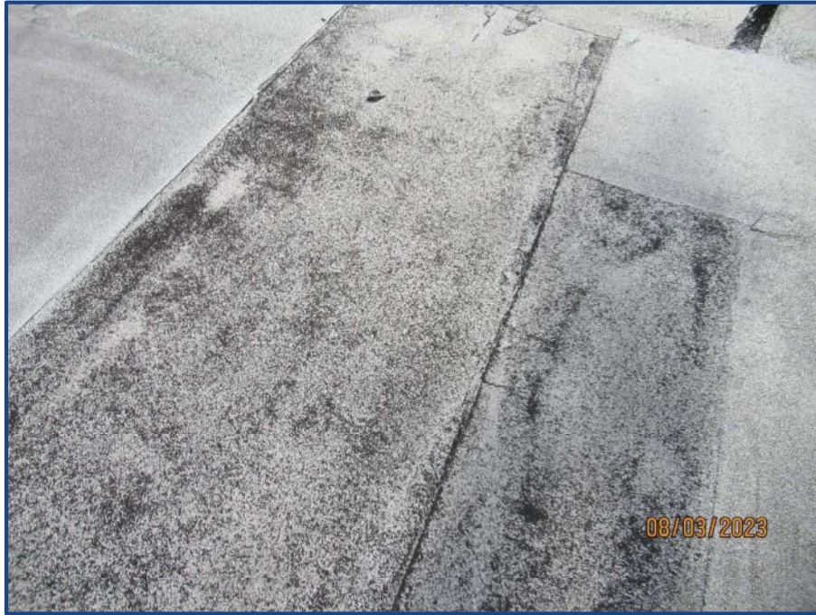
Photograph No. 17: View of granular loss and significant deterioration in the roof membrane.
