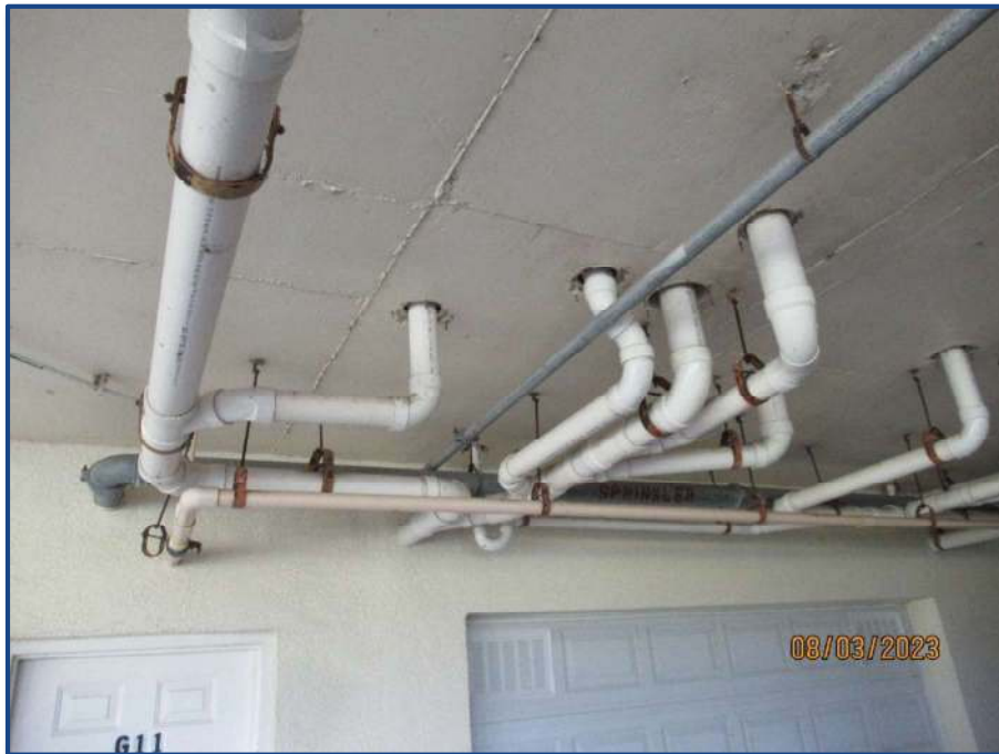
Photograph No. 32: General view of the plumbing located at the garage floor.
