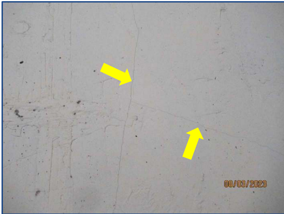
Photograph No. 20: View of cracks in the interior wall of Stair 1 Floor 5.
