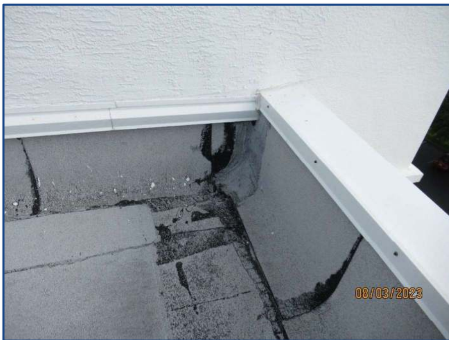
Photograph No. 16: View of granular loss and significant deterioration in the roof membrane.
