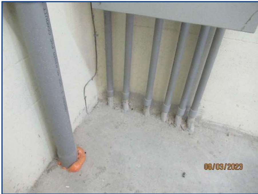
Photograph No. 38: Electrical conduits.
